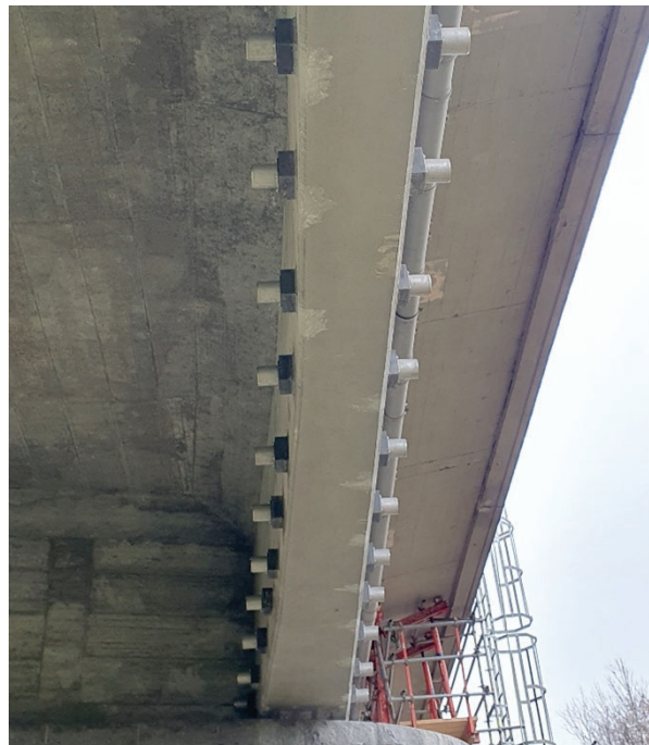
Figure 10: Hybrid anchor plates with inclination corresponding to the alignment of the existing structure
