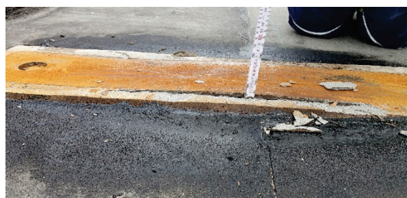
Figure 9: Distorted connection plate without a central anchor bolt after experimental heating.
