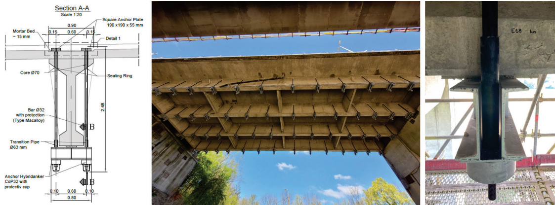
Figure 14: Cross-section of the shear strengthening ( left ); overview of the pt system ( middle ); Detail of the crossbeam with the HA plate ( right )
