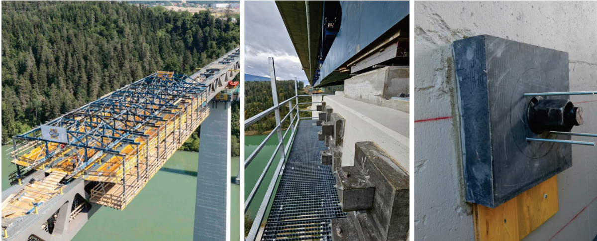
Figure 13: Construction works for the widening of the superstructure ( left ); overview of the shear strengthening with HA ( middle ); Detail of the HA plate during installation ( right )
