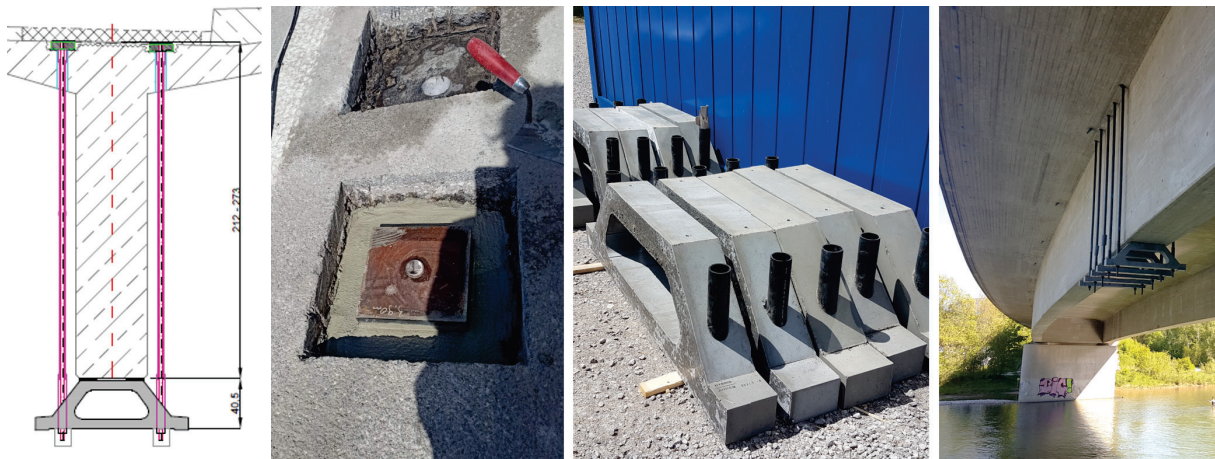
Figure 10: Drawing of the shear strengthening (1); installation of the threaded ended plates (2); CoBeam traverses before installation (3); overview of the shear strengthening from below(4)
