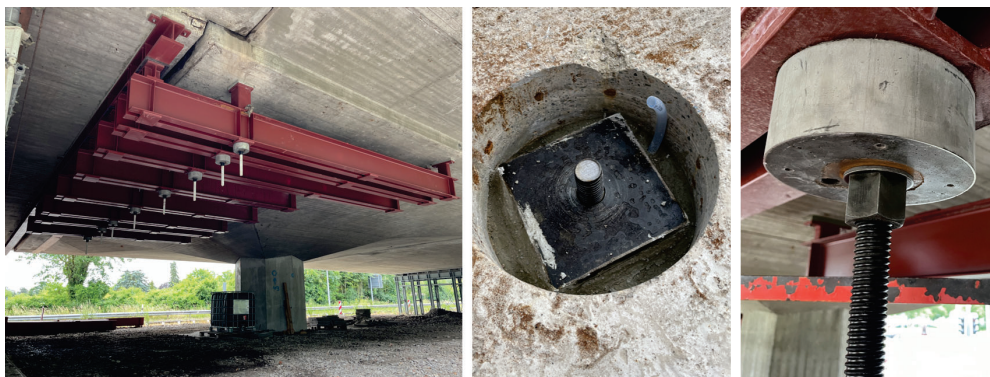
Figure 15: Overview of the strengthening system from below ( left ); Detail of the threaded ended plate on the bridge slab ( middle ); Detail of the Hybridanker plate below the steel construction ( right )
