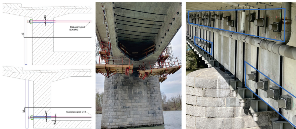
Figure 11: Cross-Section of the shear strengthening near the piers ( left ); overview of the pt system from below ( middle ); side view of the pt system with the HA plates, highlighted in the blue framed boxes ( right )
