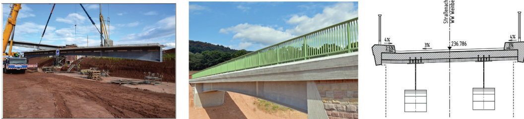
Figure 3: First hot-dip galvanized composite frame bridge in Germany over the BAB 44 motorway [21]
