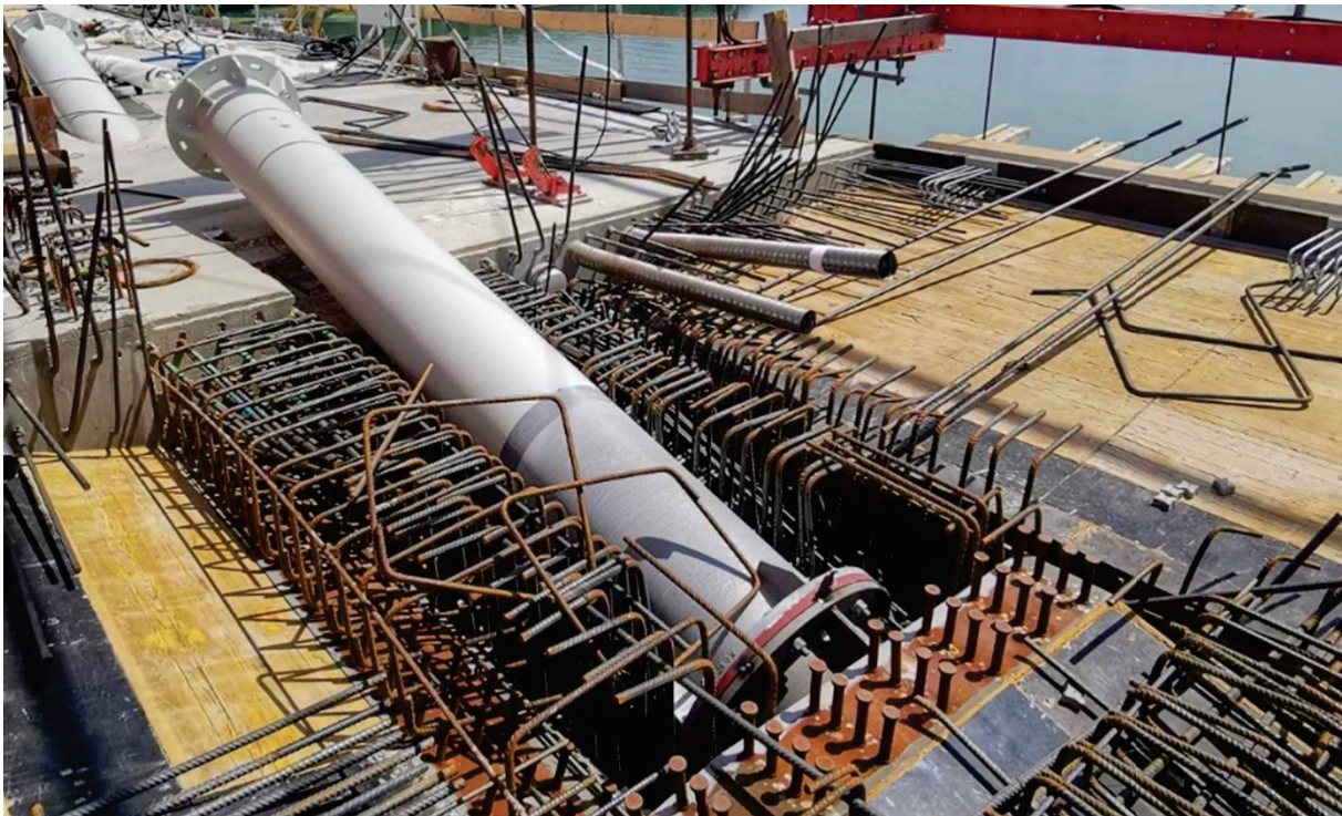
Figure 10: The extradosed cable's protection pipe to be concreted into the anchorage block
