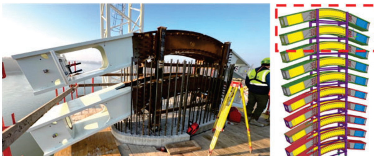
Figure 7: Fine setting of the top cable anchorage link unit (left), detailed TEKLA model of the link unit (right) – © CÉH
