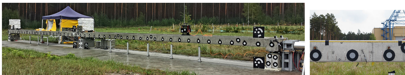
Fig. 12 Bridge example: Two span concrete test bridge at BAM testing side (left) and occurred crack pattern in the middle of the first field (right)
