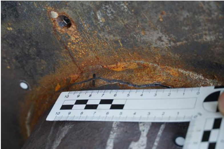
Figure 3-13 Rupture of the filled welding seam of endplate and hollow section (KR-6).
