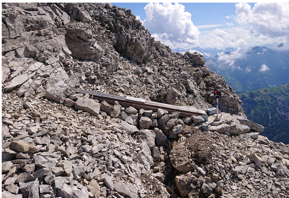
Supplementary Fig. A.1.2: Photo of vibrating wire crackmeter “Crack06” with wood roof.
