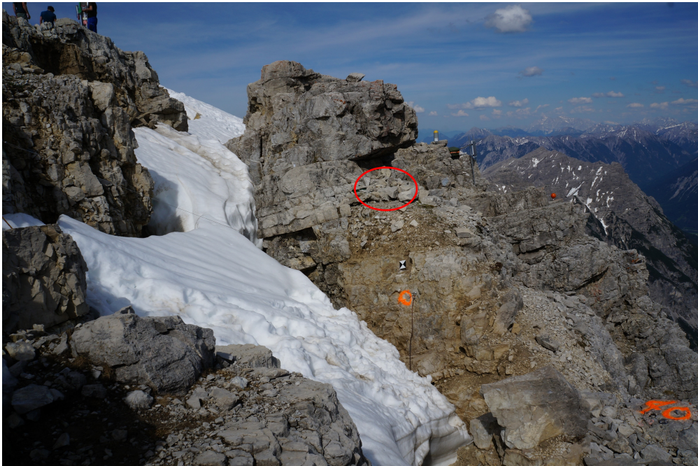
Supplementary Fig. A.1.4: Photo of the main crack with position of seismic station HV1 (red ellipse).
