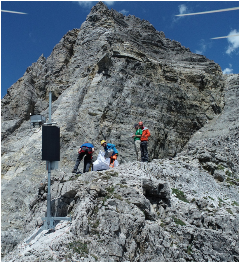
Figure 3.10: Drone photo of the installed deformation camera looking at the steep SW-wall of the Hochvogel summit. The 4 m-pole with camera, solar panel and battery is fixed to the rock mass and is grounded with copper cables.
