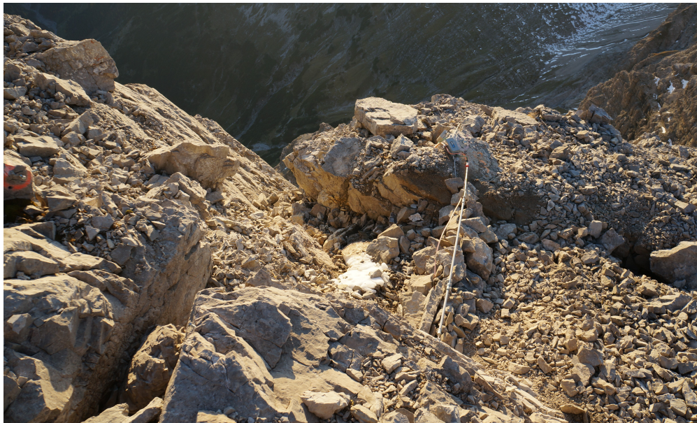
Supplementary Fig. A.1.1: Photo of vibrating wire crackmeter “Crack06” without its protective wood roof.
