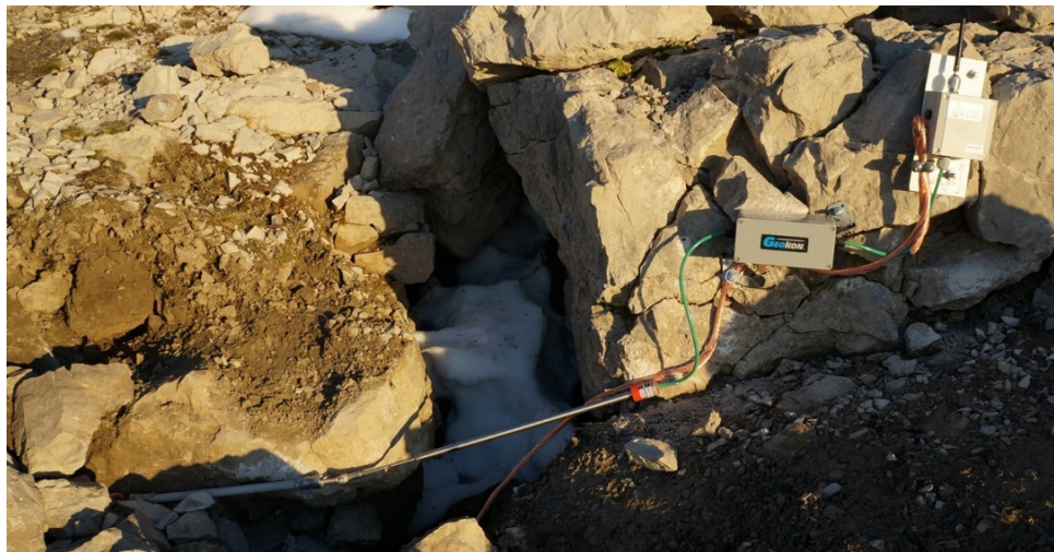
Figure 3.9: Concept of the lightning protection for crackmeters and according photo from the site (from Leinauer et al., 2021).
