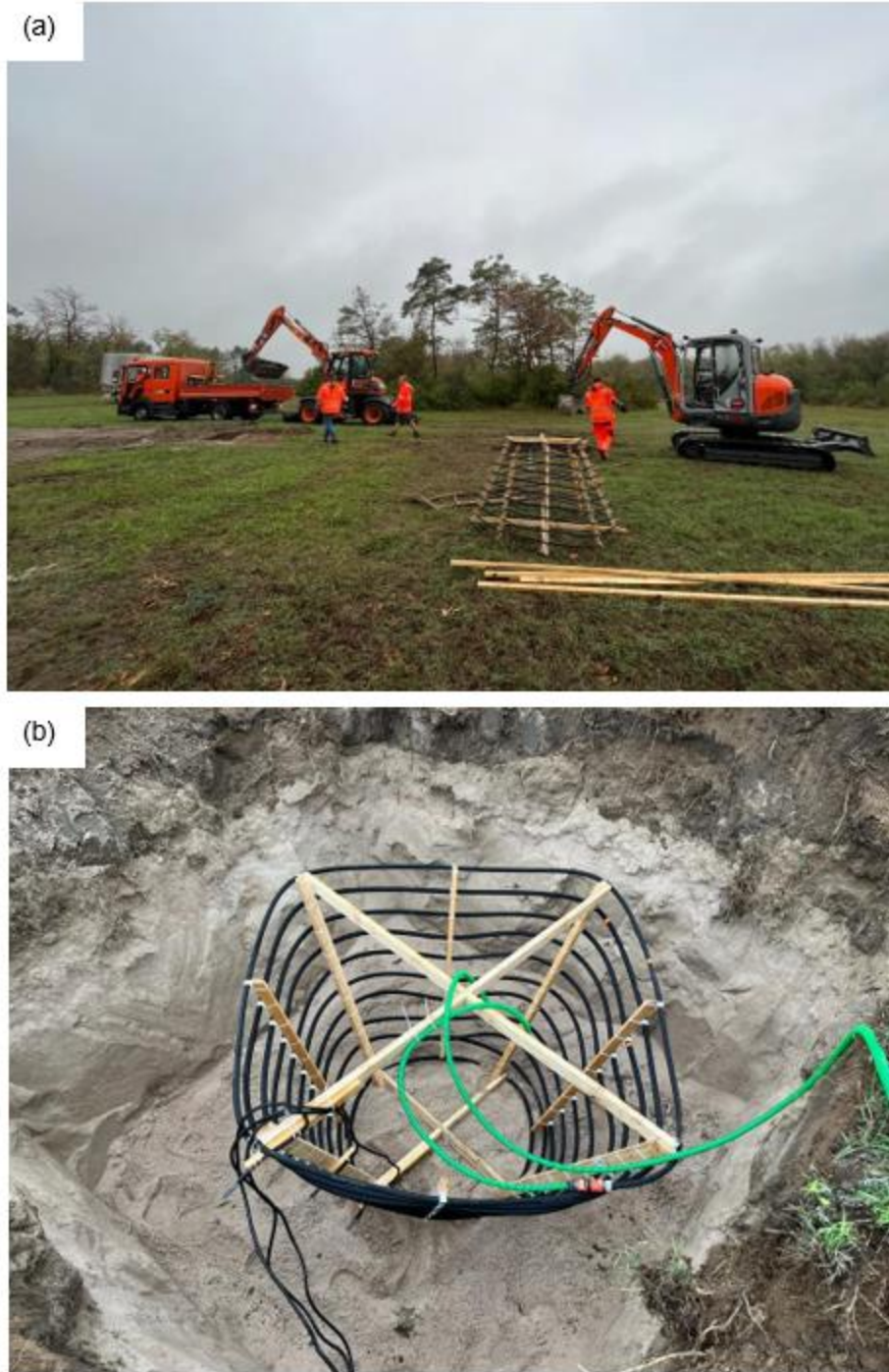
Figure 42 (a) Excavation of soil for prototypes installation (b) Installation of Prototype 1 at 1.5 m bgl.
