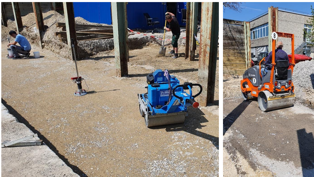
Fig. 3-10: Compaction works after placement of each soil layer using 0.4 and 1.6 t tandem rollers
