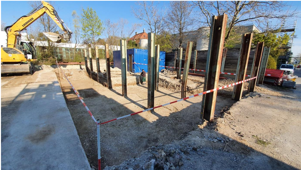
Fig. 3-9: Excavation and replacement of the soil on the testing field at Zentrum Geotechnik
