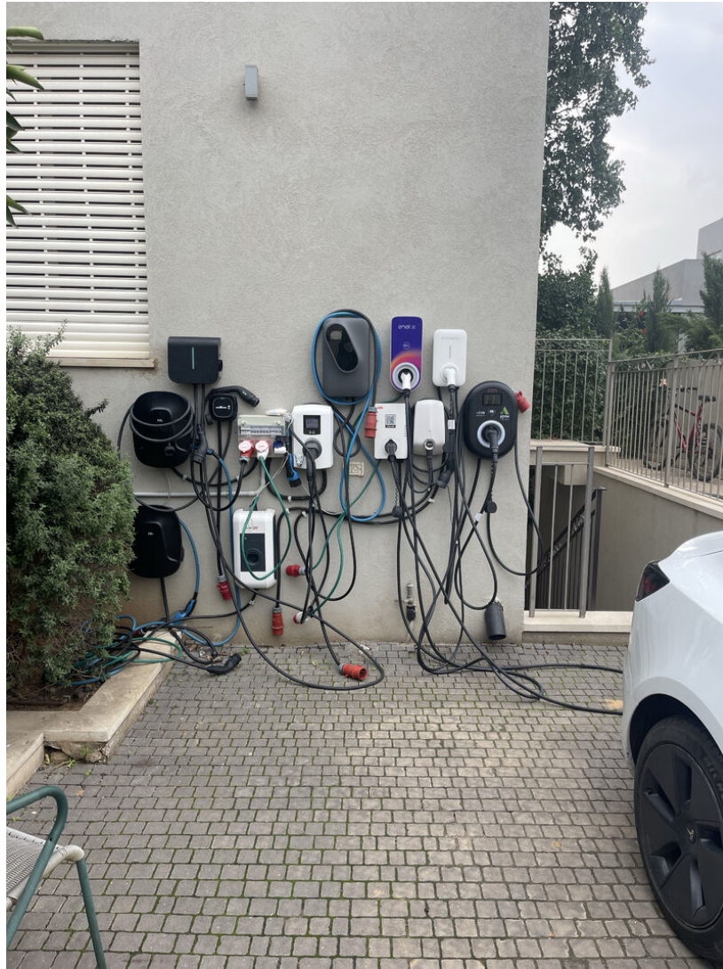
Figure 1.8 – Example of a charging station for conductive charging with bad interoperability from the infrastructure side [51].
