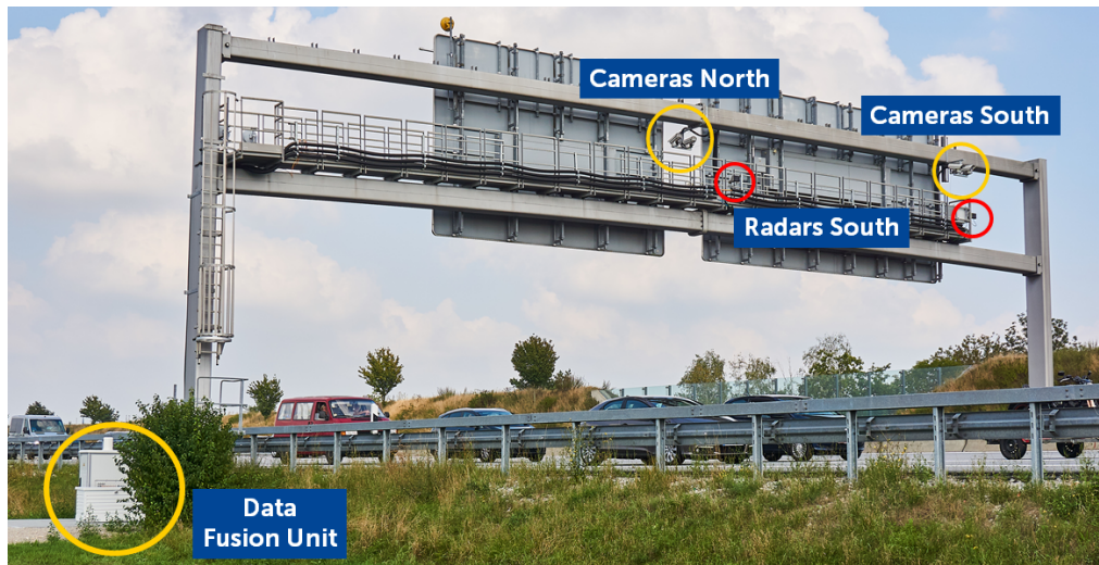
Figure 5.1: One of the Providentia measurement points on the A9 highway in Germany. The two radars directed towards the north are installed on the other side of the gantry bridge and are therefore not visible from this perspective.
