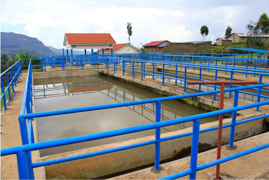
xxvi) After flocculation, the sedimentation is carried out in one of three clarifiers. Photo by Elias Okemer.
