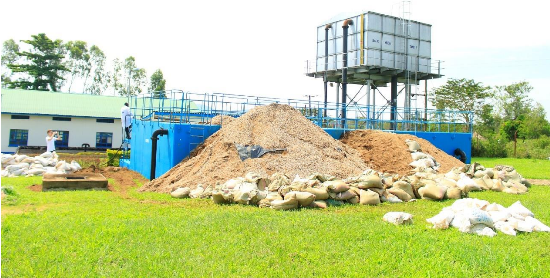
lxxiv) Overview of the maintenance works at the sand filters. Photo by Elias Okemer.
