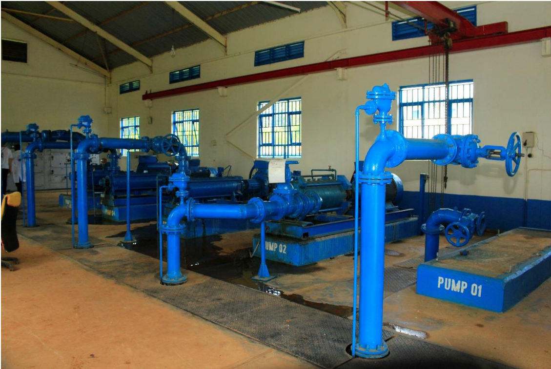
lxxxvi) Five electrical pumps transfer water from the two final water tanks (one each for the old and new line) to the reserve tank on Tororo hill. From there, the water is distributed by gravity to the water users. Two to three pumps are in operation, two to three in standby, depending on the operational conditions. Photo by Elias Okemer.
