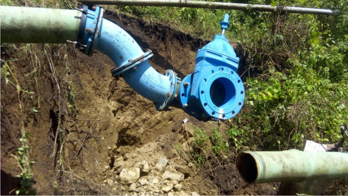
xviii) Landslides and soil movements may dislocate distribution pipes, thereby interrupting the regular operations of NWSC in the river basin. Photo by Arima Zubair Isa.
