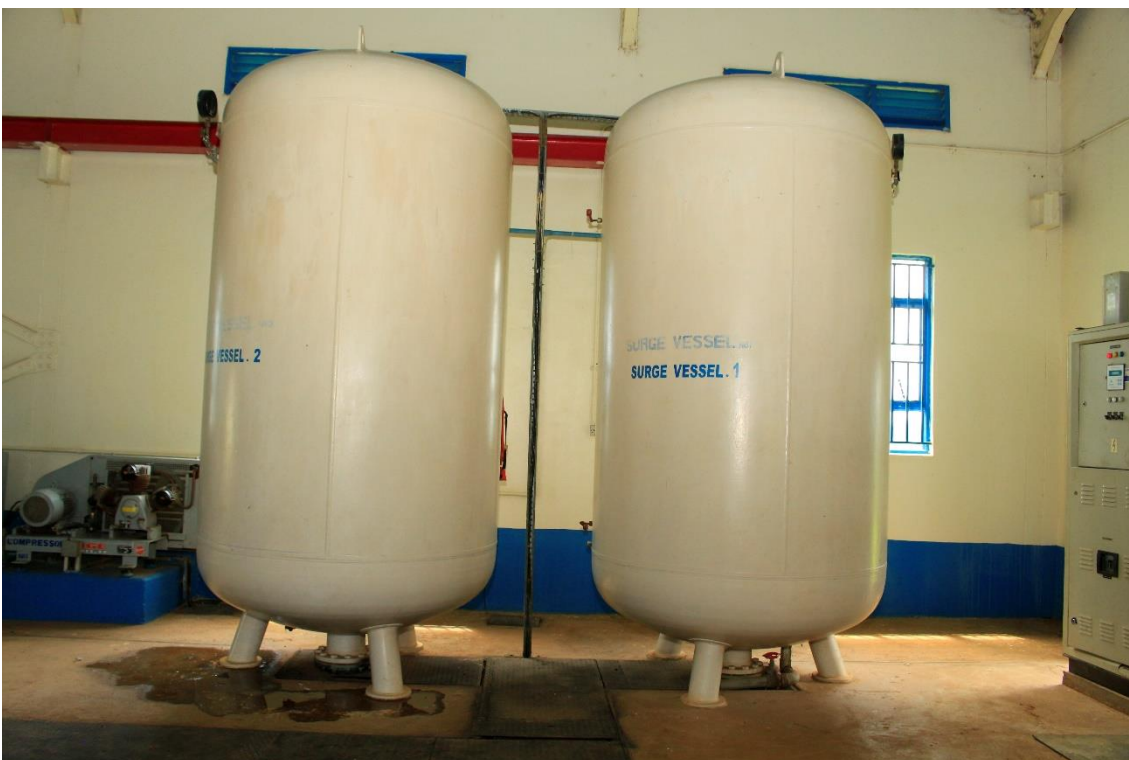
lxxxvii) Surge vessels to maintain correct pressure in the distribution network. Photo by Elias Okemer.
