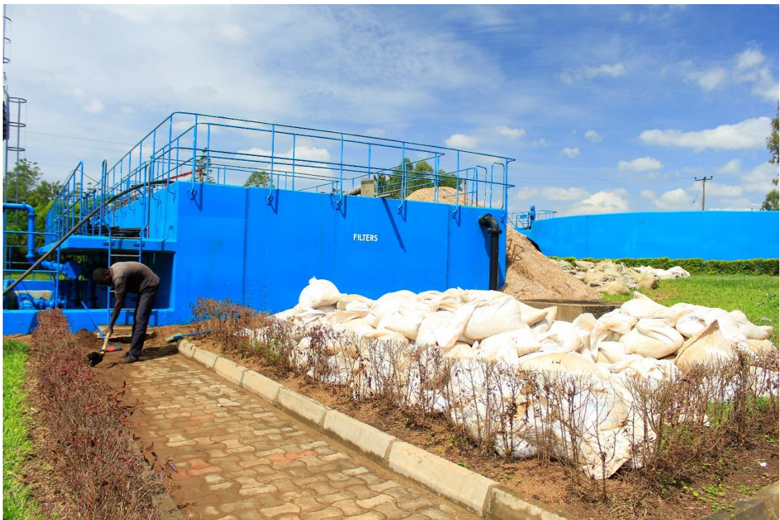
lxxiii) Sand filters at the new line. The filter media was exchanged at the time of the site visit. Photo by Elias Okemer.
