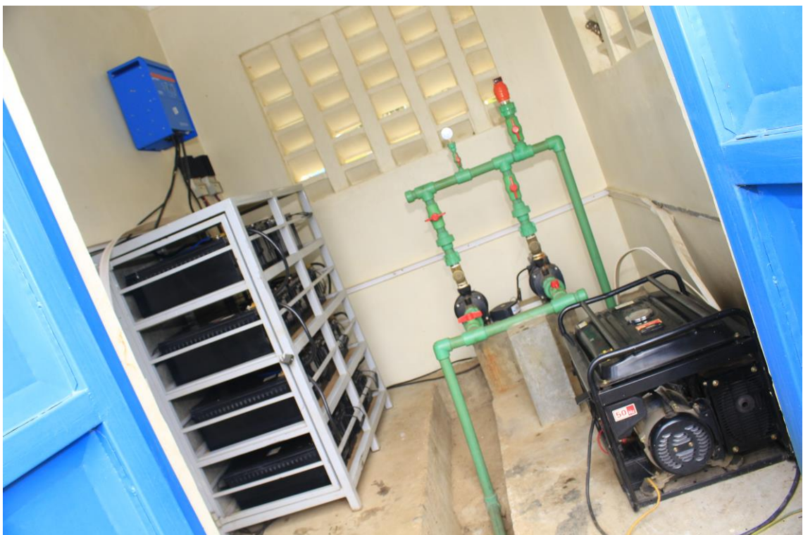
xxxiii) Interior view of the pump house. Two backwash pumps are visible in the middle of the photo, connected to green pipes. The electricity required to operate the DWTP of Lirima is provided by a solar panel (see picture xxxv), for which the corresponding solar batteries are visible on the left. A backup petrol generator is visible on the right. Photo by Elias Okemer.
