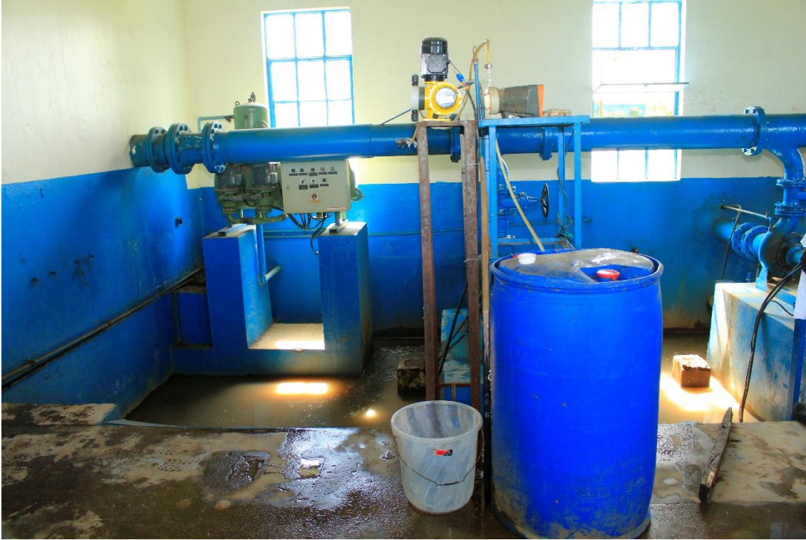
lxvi) Dosing device to apply the coagulant Aluminium Chlorohydrate (ACH) from the blue barrel to the raw water. The dosing device is operated by electrical dosing pumps. One pump is in operation, two are in standby. Photo by Elias Okemer.
