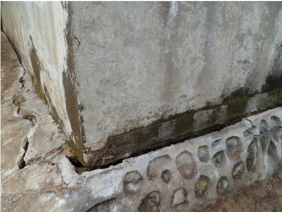
iv) Damages at the clear water well of Sono. The area is prone to land movements, resulting in frequent supply interruptions at the DWTP.
