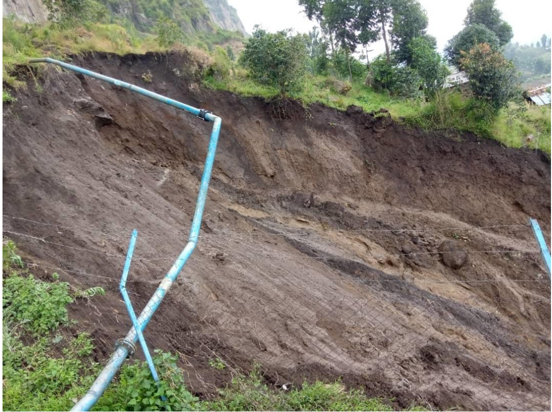
xvi) Intensive rainfalls in combination with steep slopes frequently result in landslides in the SMMRB. Thereby, large rupture surfaces are created. Often, NWSC infrastructure is affected by these natural hazards. Photo by Arima Zubair Isa.
