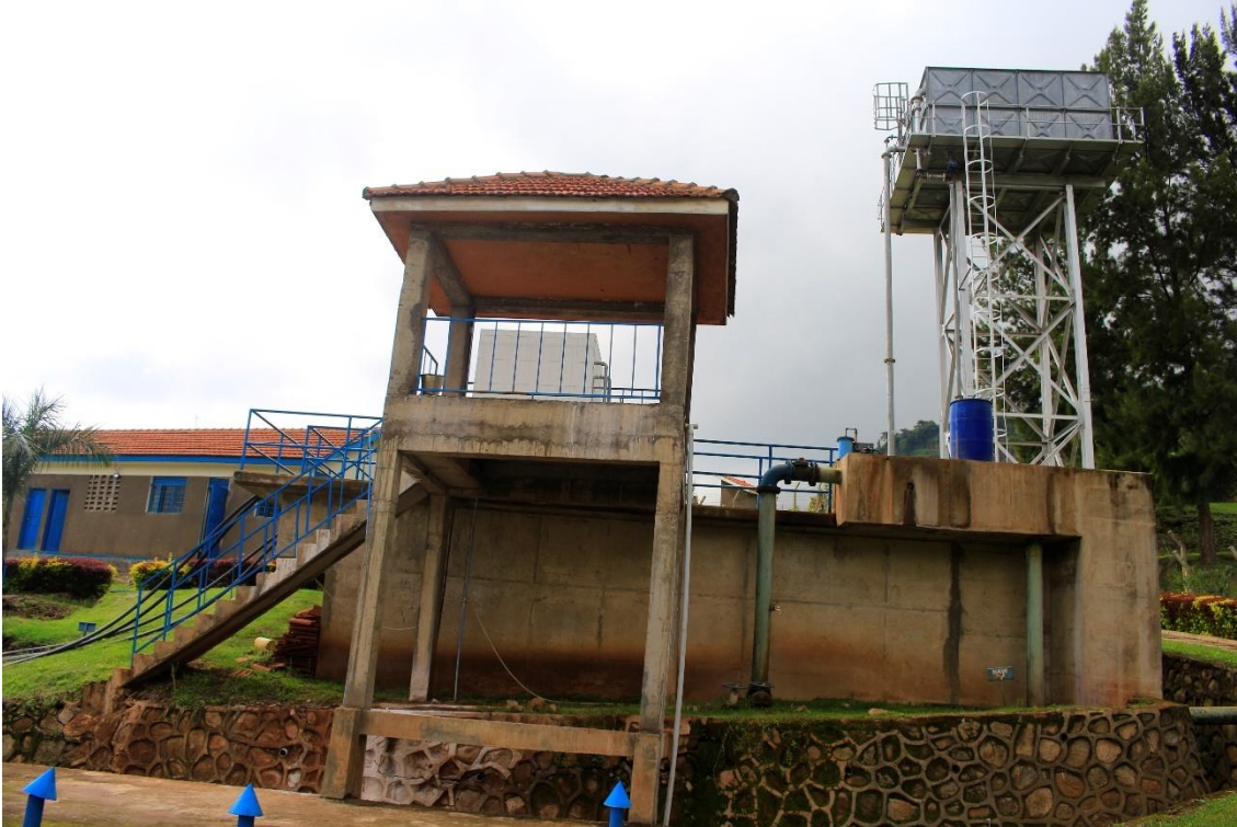
xlvi) Opposite point of view to the previous picture. The chlorine tank for disinfectant dosing is located under the roof, behind it the clarifiers for sedimentation. Elevated backwash water tank on the right. The blue barrel on the right is the alum drum facilitating coagulant dosing to the raw water. In the background is the plant building including the office, laboratory, storage spaces, etc. In the lower part is the clear water well for the final water. Photo by Elias Okemer.
