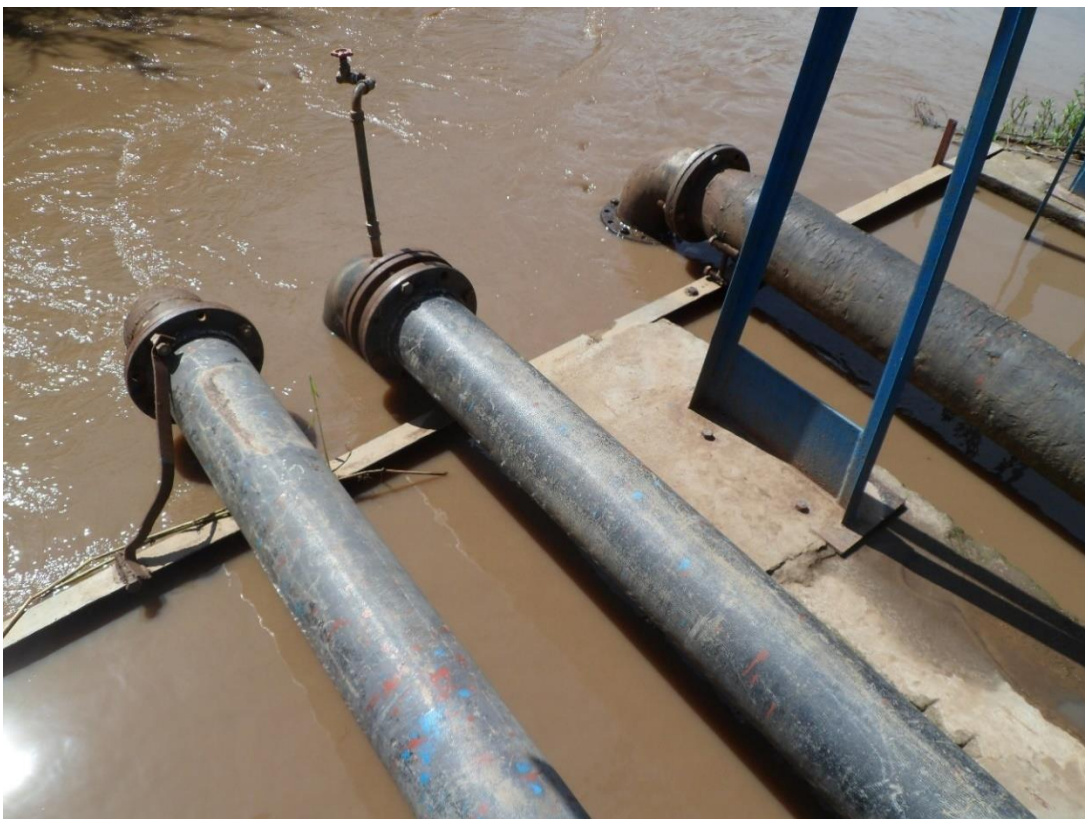
lxiii) Raw water intake pumps of Malaba-Tororo. Three pipes are visible on the water surface, another pump is located under water. When the intake pipes get too clogged due to sediment deposits, the corresponding pumps are shut off to allow for the sediment to be flushed away by the turbulent stream water. After a while, the pumps can be turned on again and operation can continue. Furthermore, a diver removes sediments regularly.
