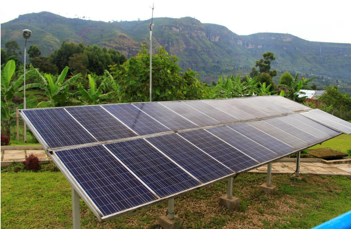
xxxv) Solar panel providing electricity for the operation of Lirima. Photo by Elias Okemer.
