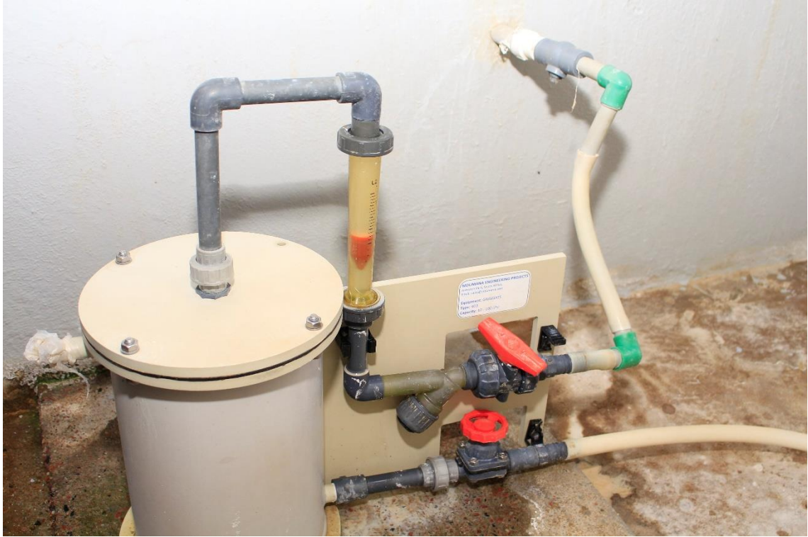
xxiv) A gravity-operated dosing device doses the coagulant solution from the alum tank to the raw water. Photo by Elias Okemer.
