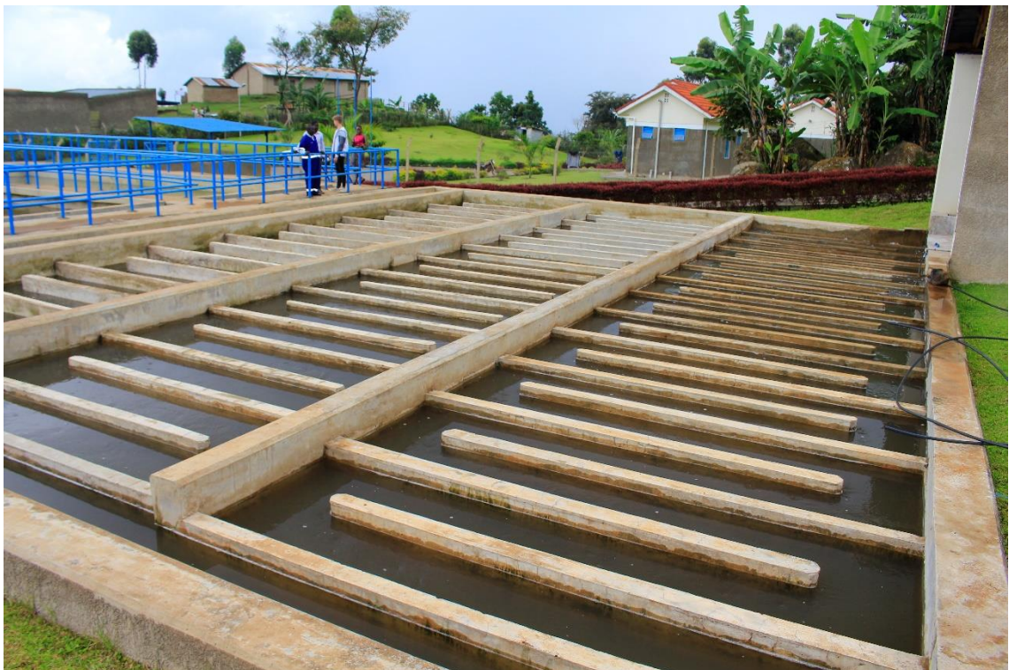
xxv) After dosing of the coagulant, the water flows into flocculation weirs. The hydraulic flocculation system ensures the required mixing and turbulence, as well as sufficient flocculation time. Photo by Elias Okemer.
