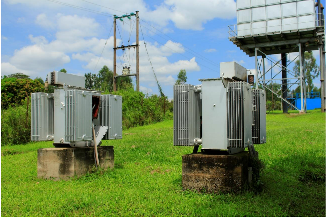
lxxxviii) The electricity required to operate the DWTP of Malaba-Tororo is provided by electricity from the grid, as well as a backup diesel generator. For the former, the photo shows the transformers, and the electricity grid in the background of the picture. Photo by Elias Okemer.
