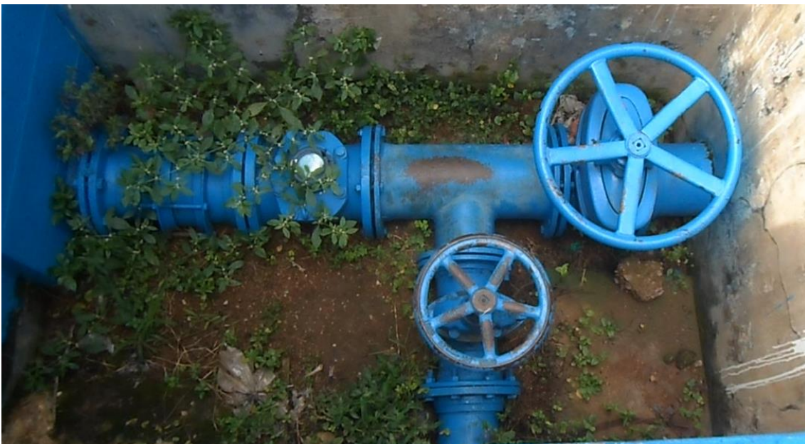
lxxix) Service water meter and control valves for the backwash water. The junction allows to feed the elevated backwash water tanks from both the new and old line with final water from the clear water well.
