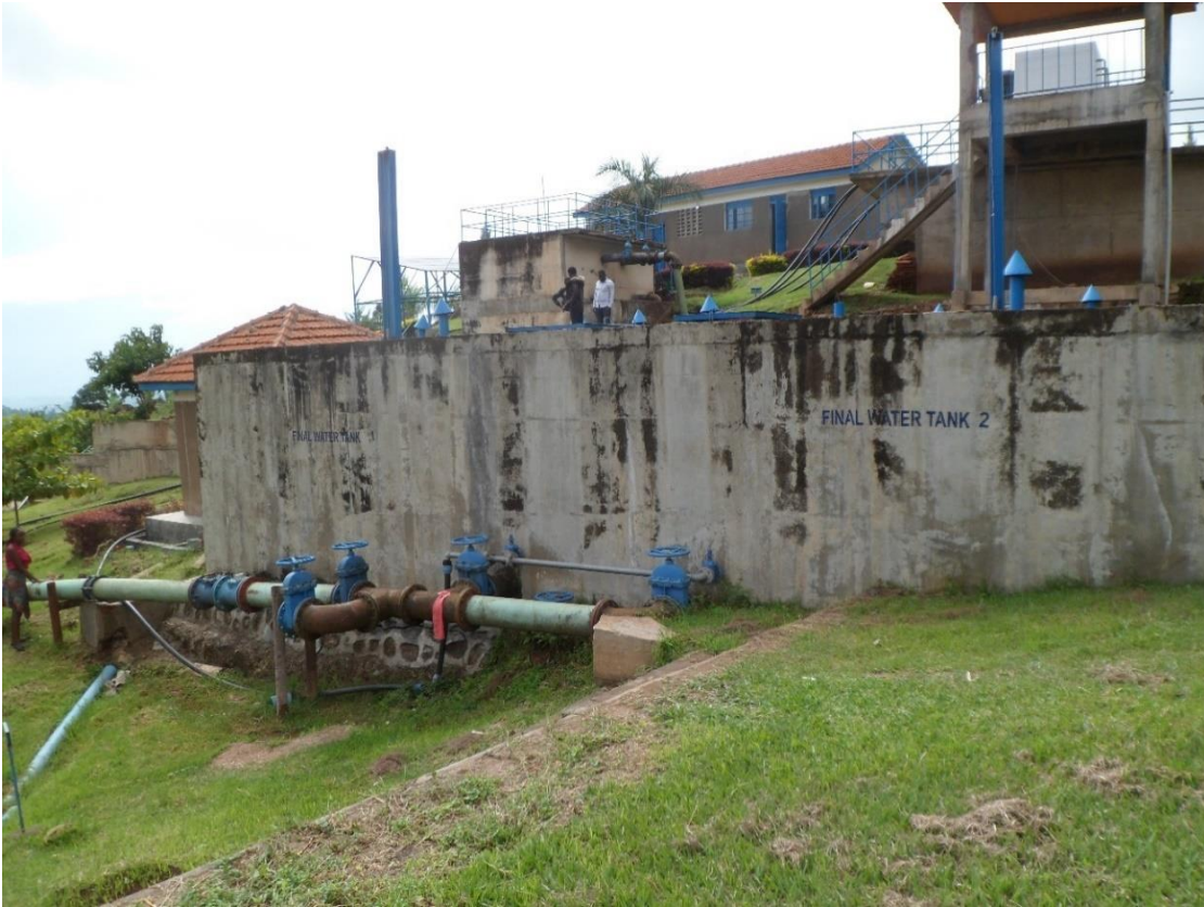
liv) Clear water well and distribution pipe, including valves to steer the outflow into the supply network.
