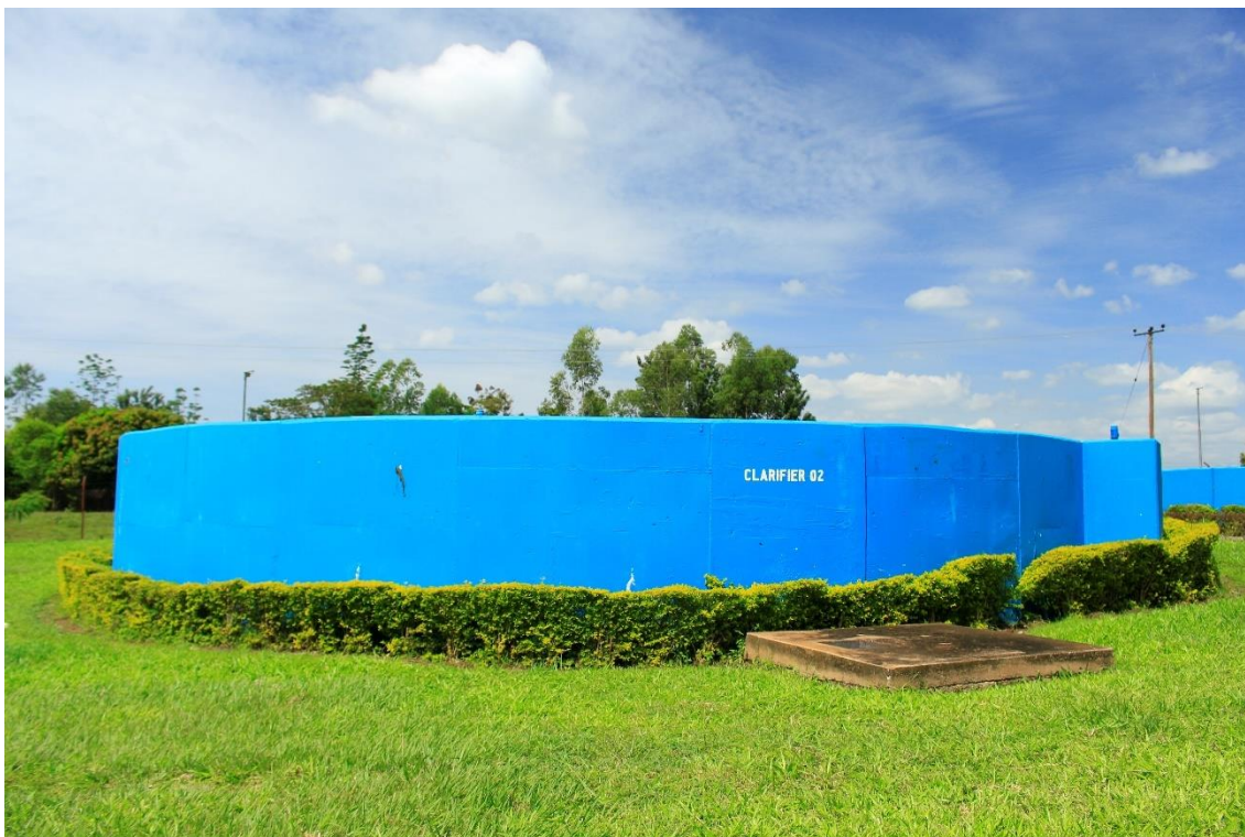
lxxi) Sedimentation basin. Two clarifiers are operated in parallel at the new line. Photo by Elias Okemer.
