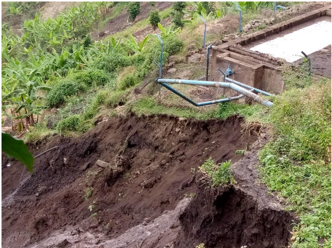
xvii) Rupture surface after a landslide event. The landslide occurred close to treatment plant buildings of NWSC. Photo by Arima Zubair Isa.
