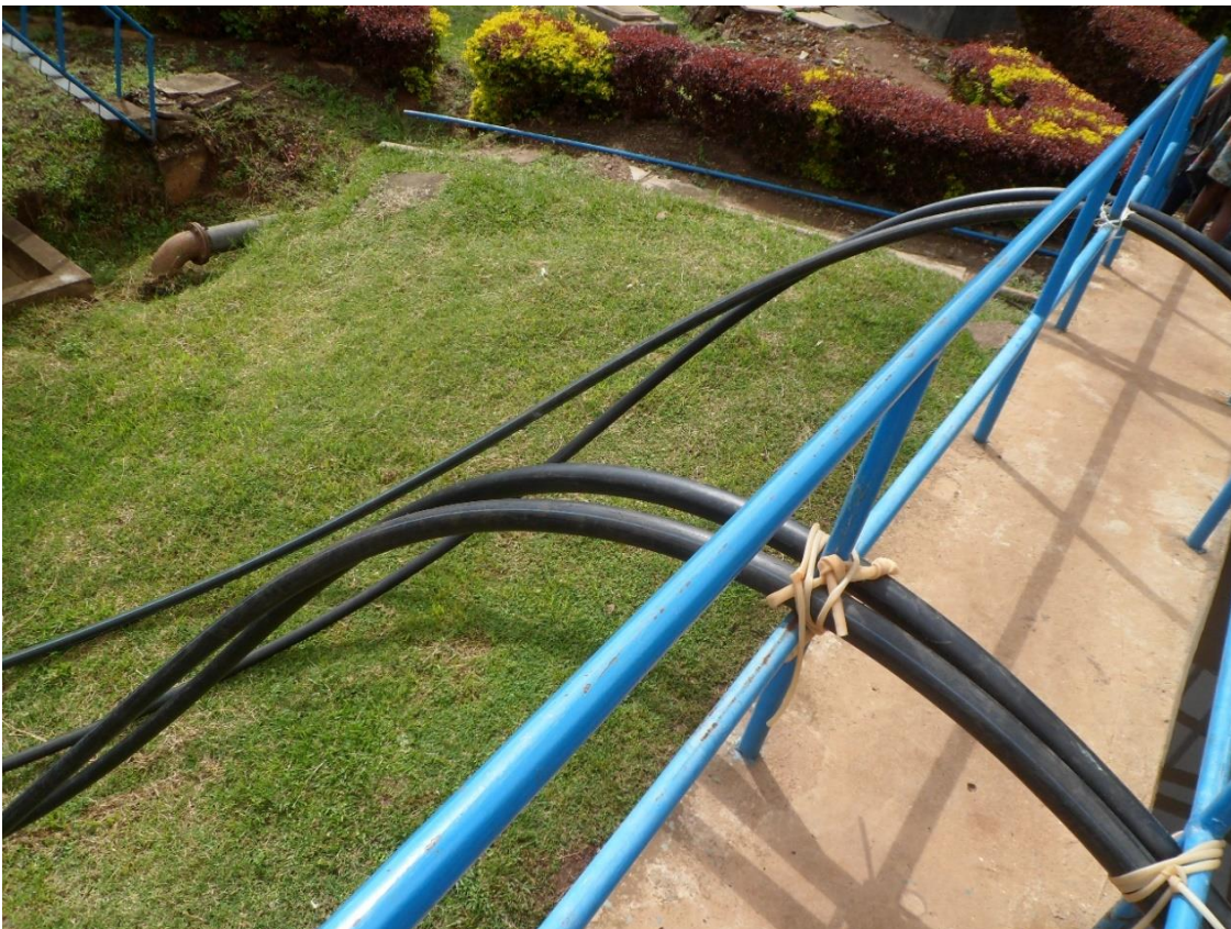
ii) As the filtration stage was not in operation as well at the time of the site visit, the raw water from the clarifiers was taken up by these tubes, bypassing the filter, and transferred directly to the clear water well.
