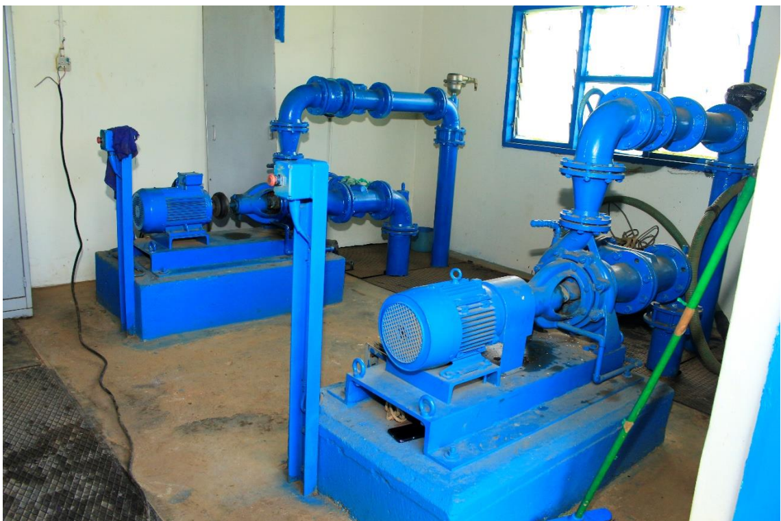
lxxvii) Interior view of the backwashing station. Two electrical pumps transfer water from the clear water wells to the backwashing tanks. One pump is in operation, one in standby. Photo by Elias Okemer.
