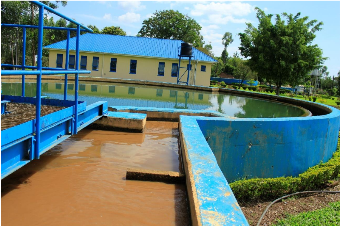
lxxii) After flocculation that took place in the raw water pipe, dense flocs can be observed in the front part of the clarifier. The flocs settle quickly, resulting in less turbid water in the rear part of the clarifier. The clarifiers need to be cleaned from sediments approximately every three months. Photo by Elias Okemer.
