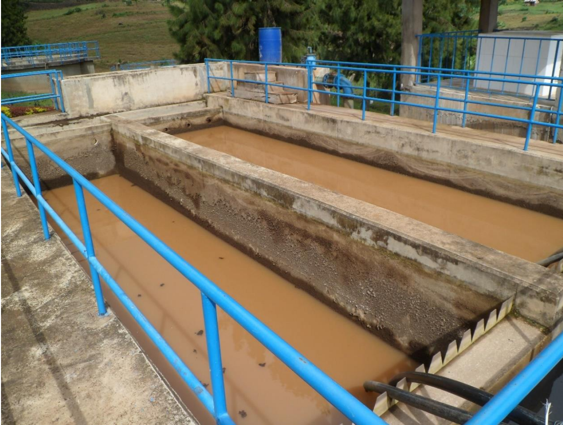
i) Both clarifiers were not in operation at the time of the site visit. Photo by Elias Okemer.
