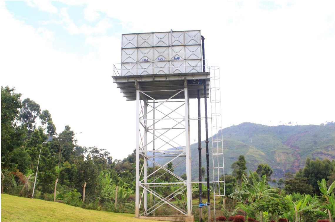
xxviii) To backwash the filters, the plant has an elevated backwash water tank. Finished water is withdrawn from the clear water well and pumped by backwash pumps to the elevated tank. During backwashing, water flows by gravity from the backwash water tank to the sand filters. Photo by Elias Okemer.
