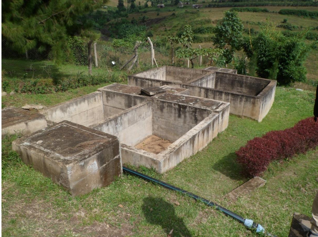
ix) Drying beds for the treatment of wastewater generated during drinking water production, mainly from backwashing and cleaning of clarifiers. The drying beds were not in operation at the time of the site visit.
