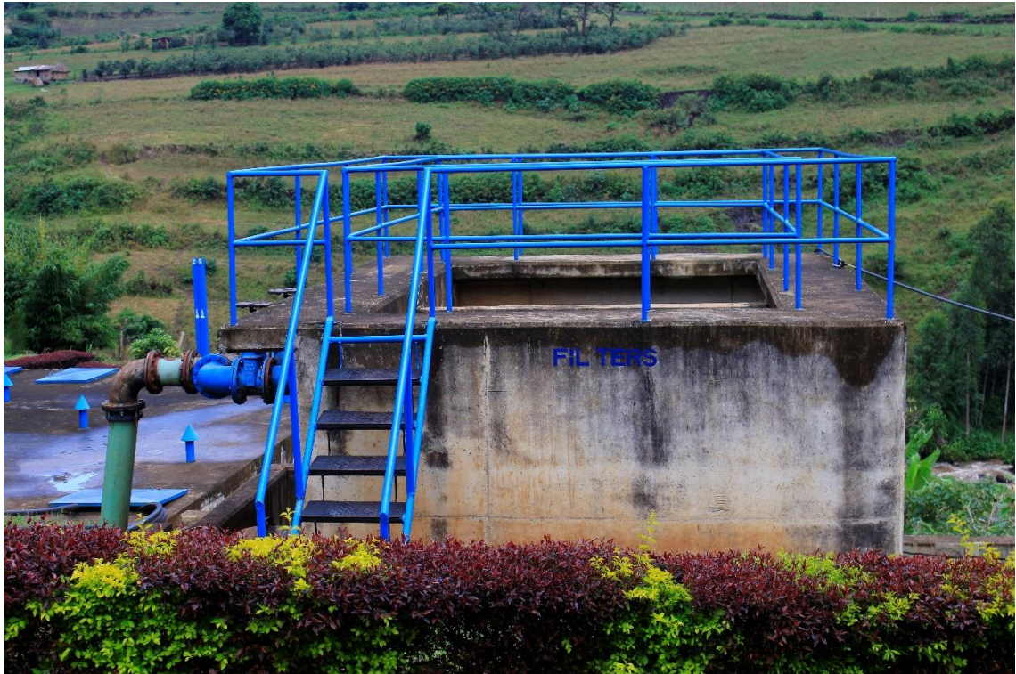
lvi) Rapid sand filters. The treatment stage was not in operation at the time of the site visit and instead bypassed by the tubes shown in picture liv. Photo by Elias Okemer.
