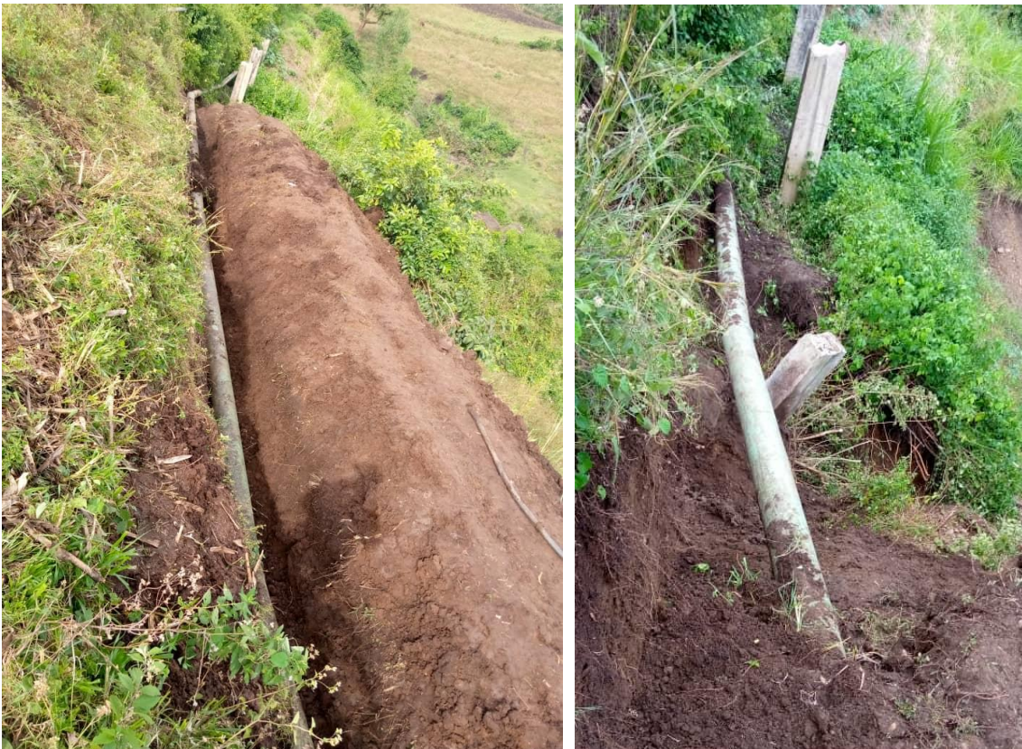
xv) Soil movements regularly affect NWSC infrastructure in the SMMRB. Photo by Arima Zubair Isa.
