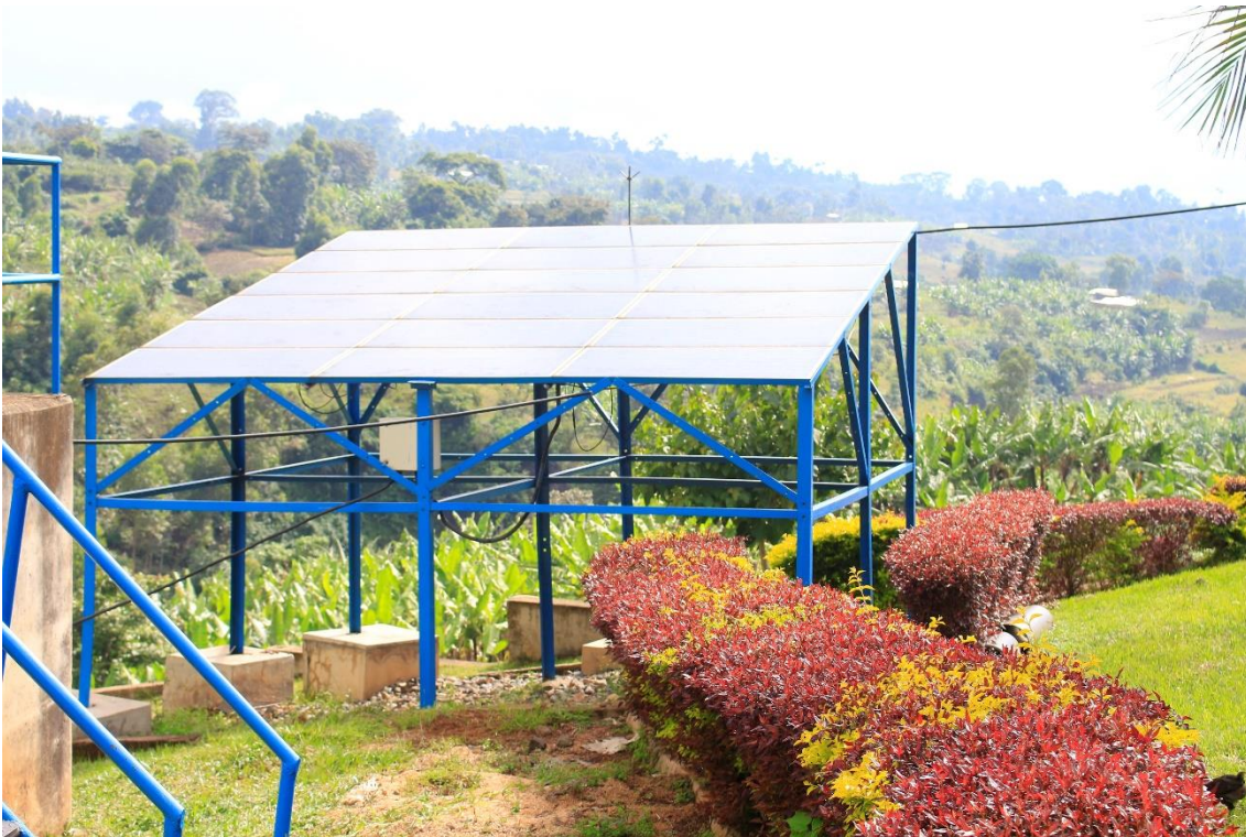
lviii) Solar panel providing electricity for the operation of Sono. Photo by Elias Okemer.
