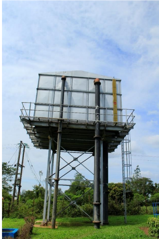
lxxx) Elevated backwashing water tank of the new line. In backwashing mode, water flows by gravity from the elevated tanks to the sand filters. Simultaneously, air is supplied by the air backwash blowers. Photo by Elias Okemer.
