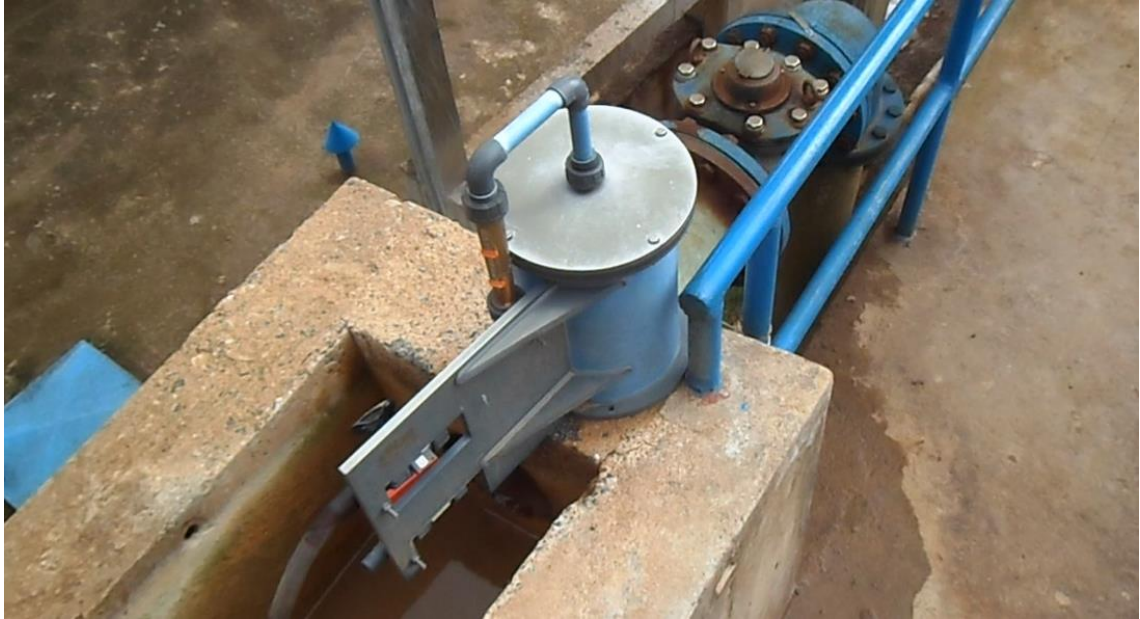
xlviii) A gravity-operated dosing device doses the coagulant solution from the alum drum to the raw water.
