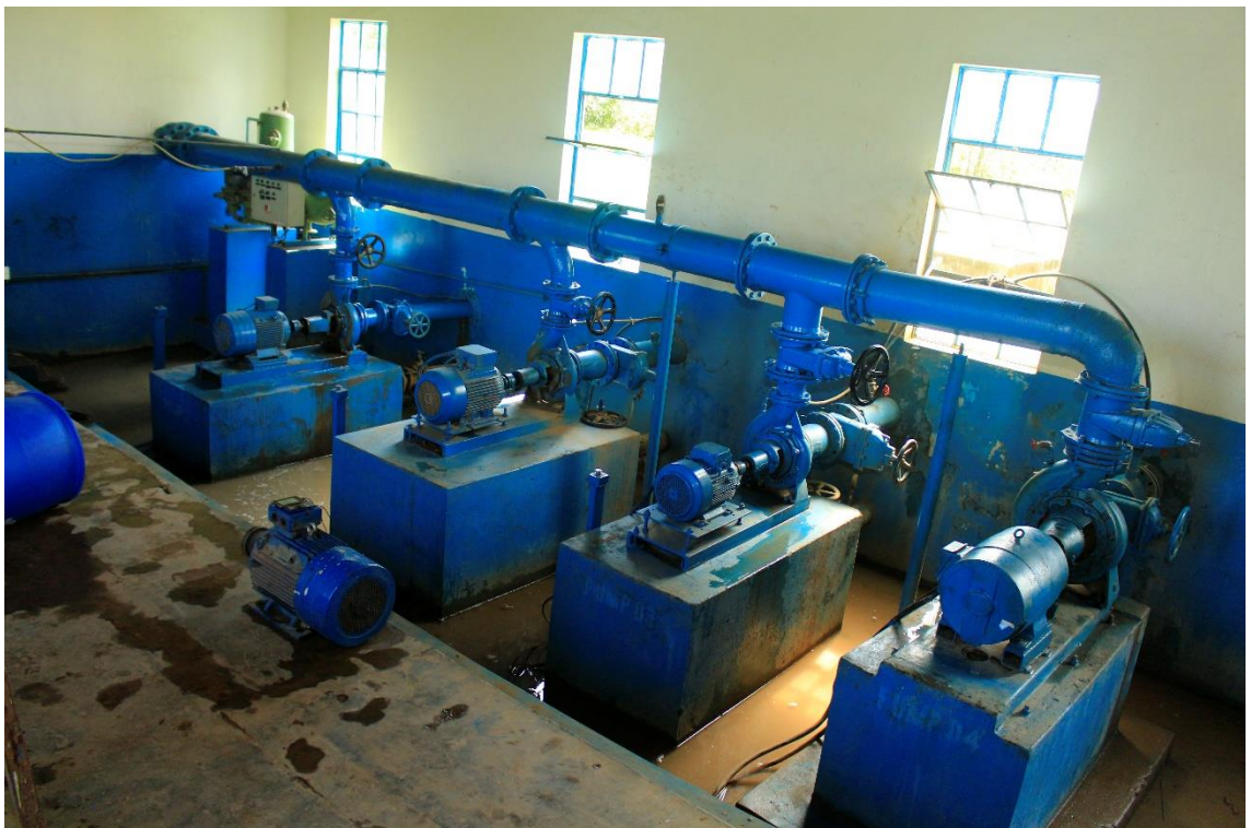
lxv) The raw water pumps draw water from river Malaba in and transport it to the DWTP. Two pumps are in operation, two in standby. Photo by Elias Okemer.
