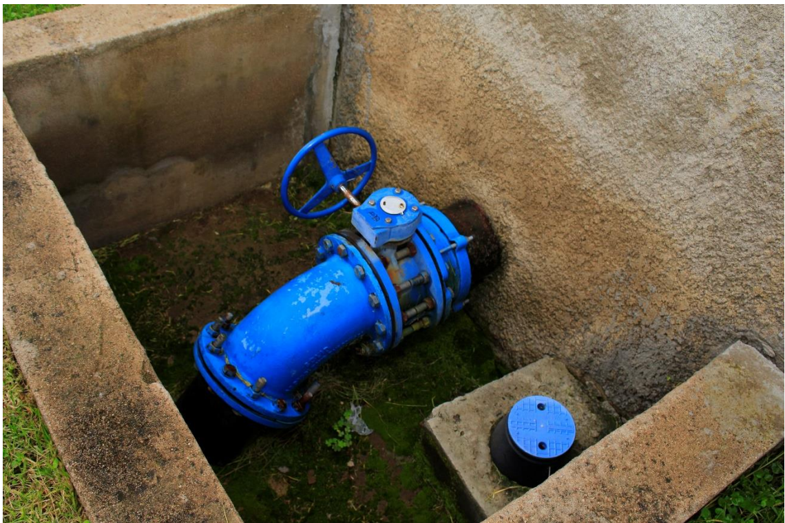
xxix) Control valve for backwash water and service water meter. Photo by Elias Okemer.
