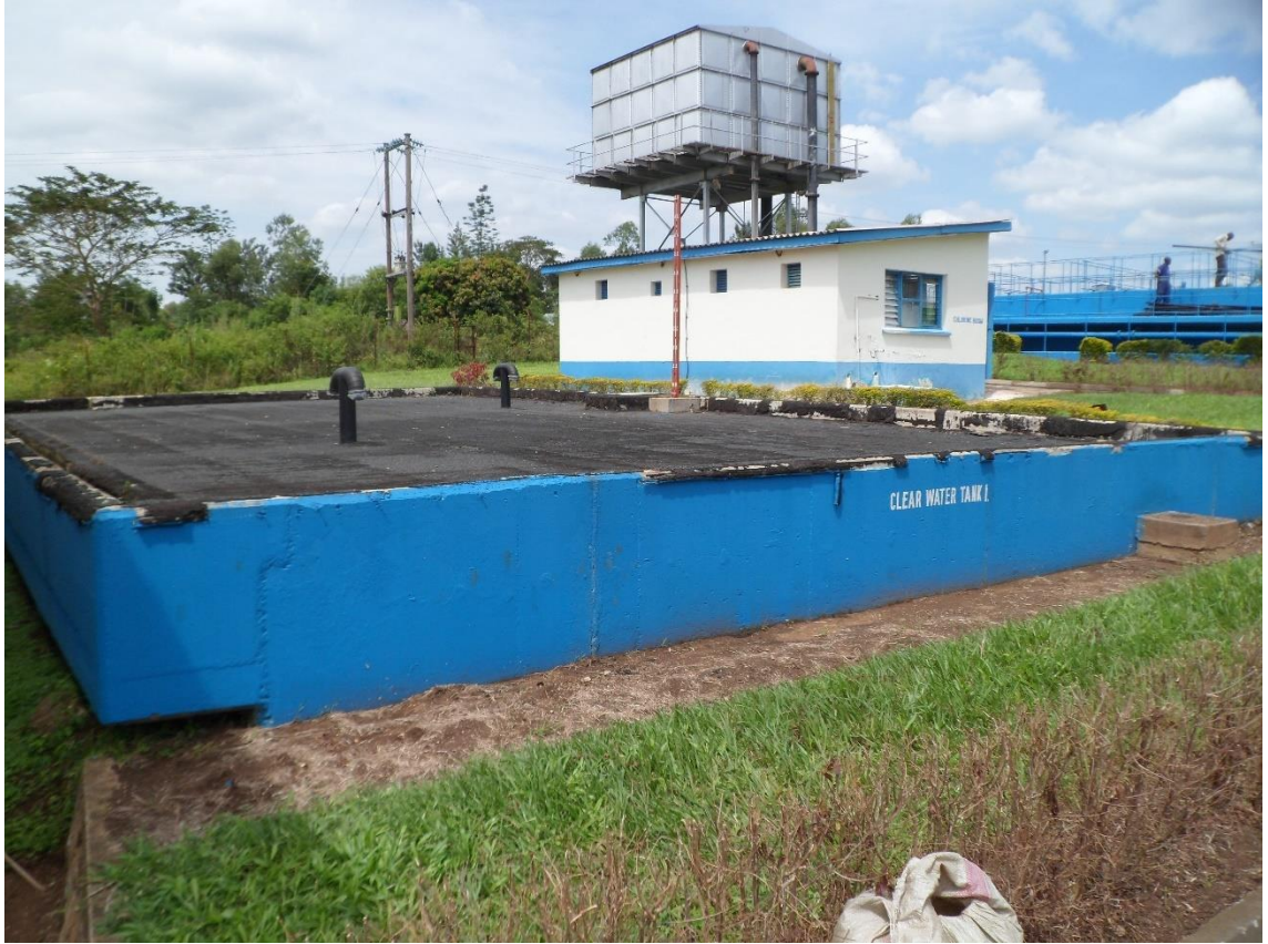
lxxxiv) Final water tank with water level meters.
