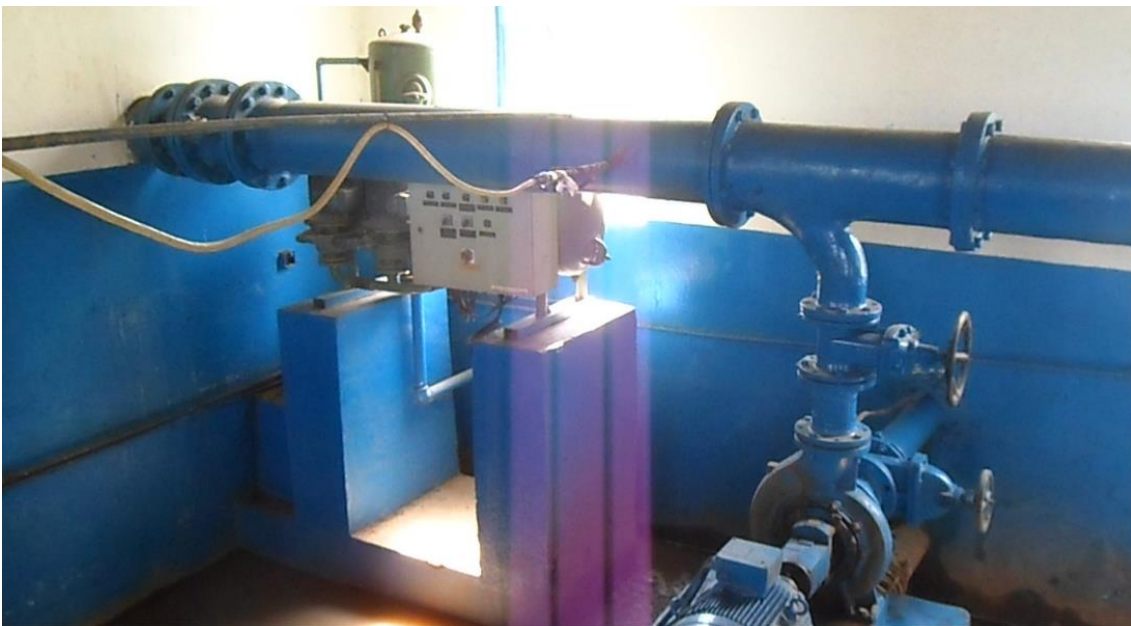
lxvii) The dosing device applies the coagulant chemical through a hose into the raw water pipe. Due to turbulence in the pipe, the coagulant is rapidly mixed with the raw water. Simultaneously, the water stream is transported to the DWTP.
