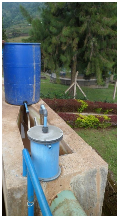
xlvii) Alum mixing drum and coagulant dosing device. In the alum drum, a sack containing alum is brought into contact with water. The alum solution flows out from the tank through a tube and is dosed to the raw water by the dosing device.
