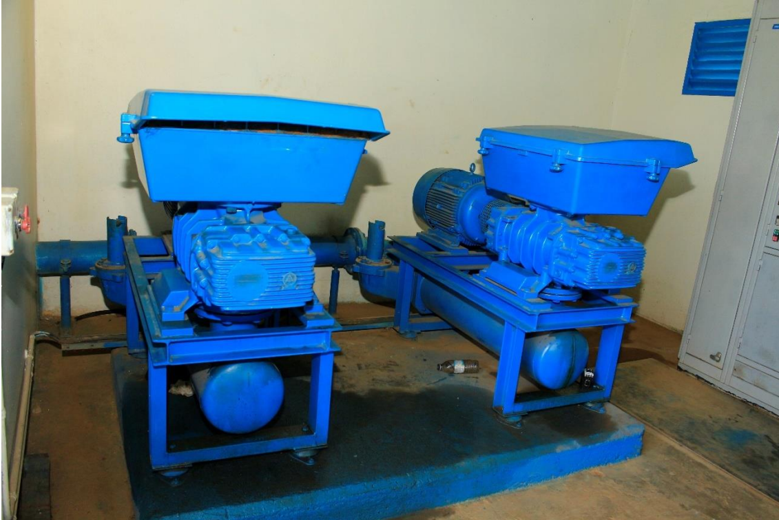
lxxviii) Air backwash blowers to provide air to the filters during backwashing. Photo by Elias Okemer.
