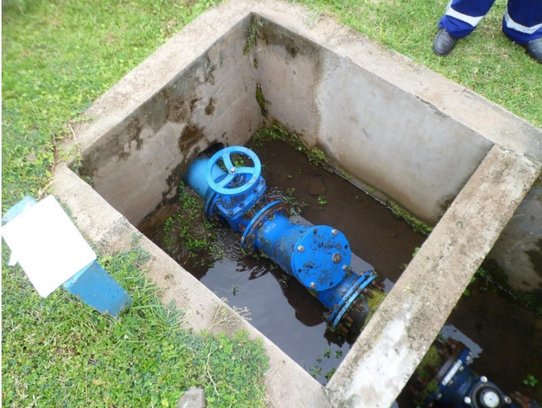
xxii) Raw water meter to assess the water quantities flowing into the plant. The corresponding plant records were evaluated as part of the present thesis.
