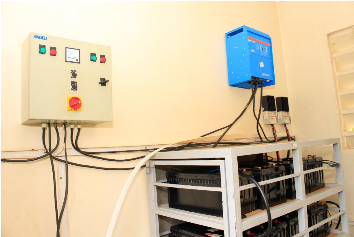
xxxiv) Interior view of the pump house. Inverter by the manufacturer Victron energy on the right. Photo by Elias Okemer.
