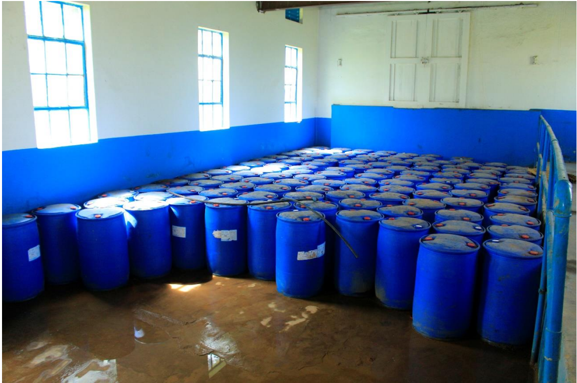
Ixviii) Storage room for ACH in the pump house. About two barrels per day were used in average at the time of the site visit, at a stock of about 130 barrels. Photo by Elias Okemer.
