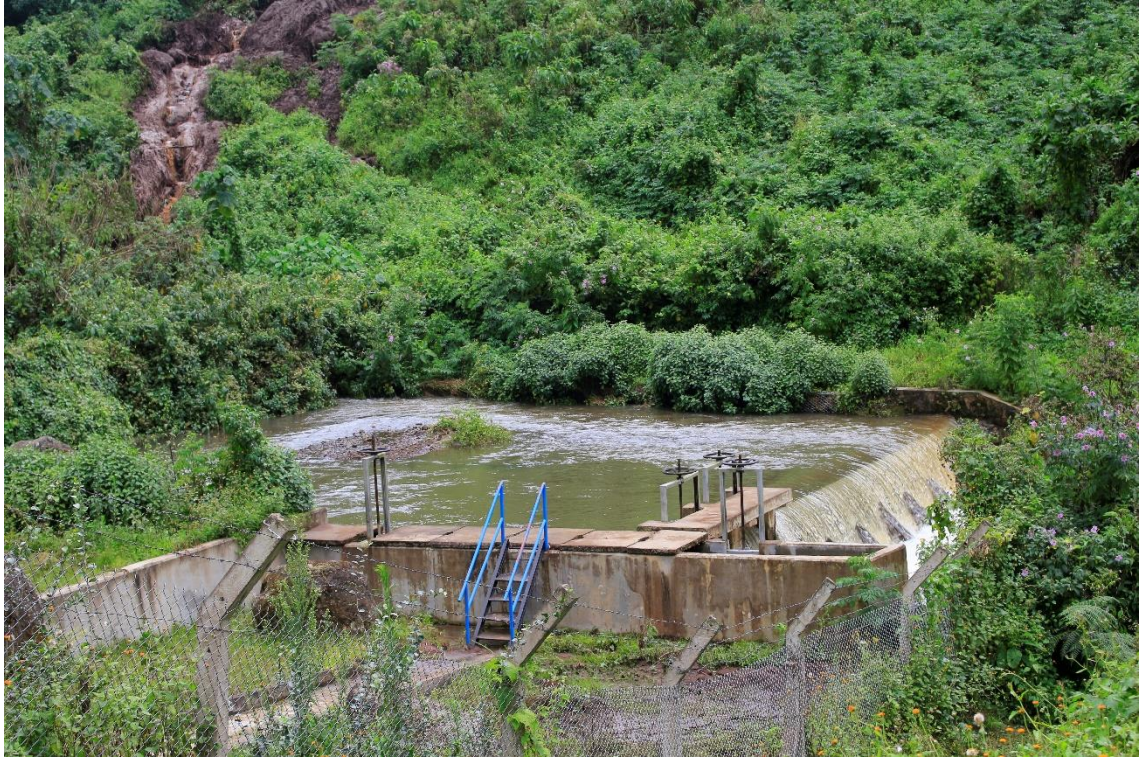
xx) The intake structure includes a weir for constant level heights, and valves to steer the inflow of raw water to the DWTP. The water flows to the plant by gravity, no raw water pumps are required. Photo by Elias Okemer.
