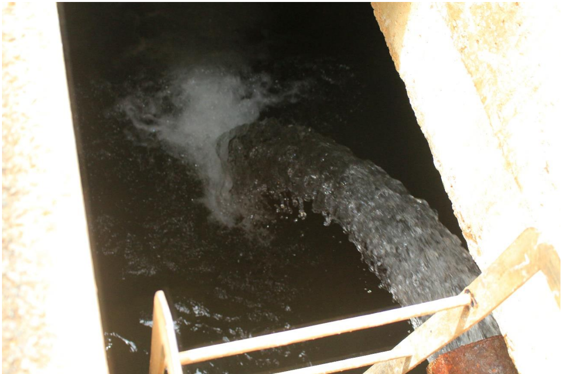
lxxxv) Interior view of the final water tank. Photo by Elias Okemer.
