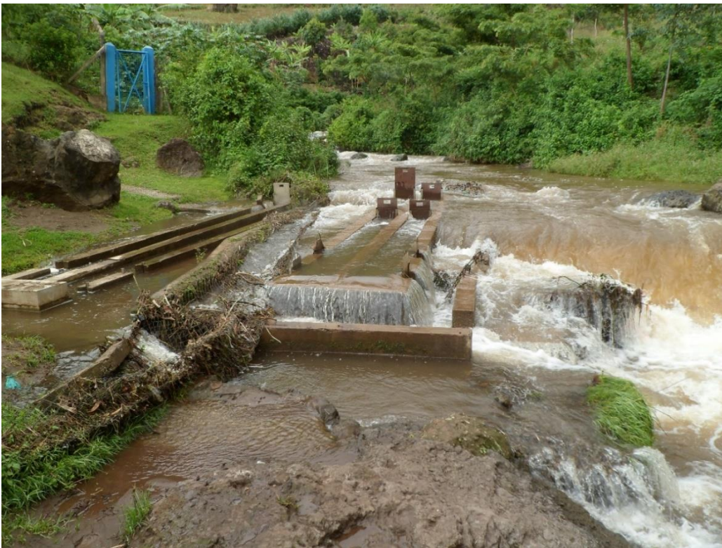
xliii) Intake structure of Sono Gravity Flow Scheme. The intake of the new DWTP which is in operation today is visible in the middle of the picture. On the left is the former intake structure of the old plant which is no longer used today.
