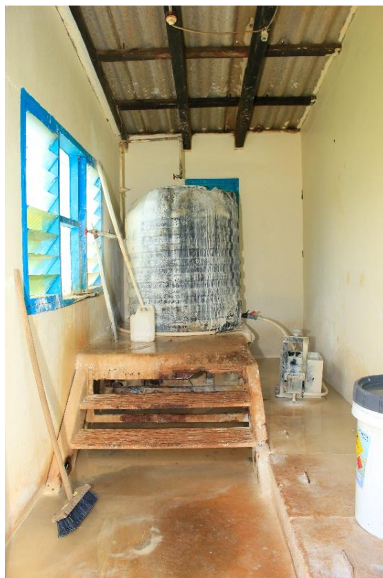
lxxxi) Chlorine tank and dosing device in the chlorine room. Photo by Elias Okemer.
