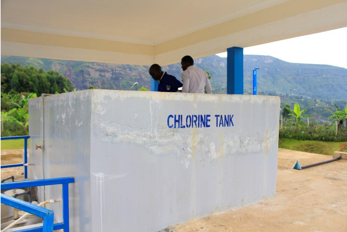
xxx) In the chlorine tank, the disinfectant solution is prepared and stored before it is dosed to the water stream. Photo by Elias Okemer.
