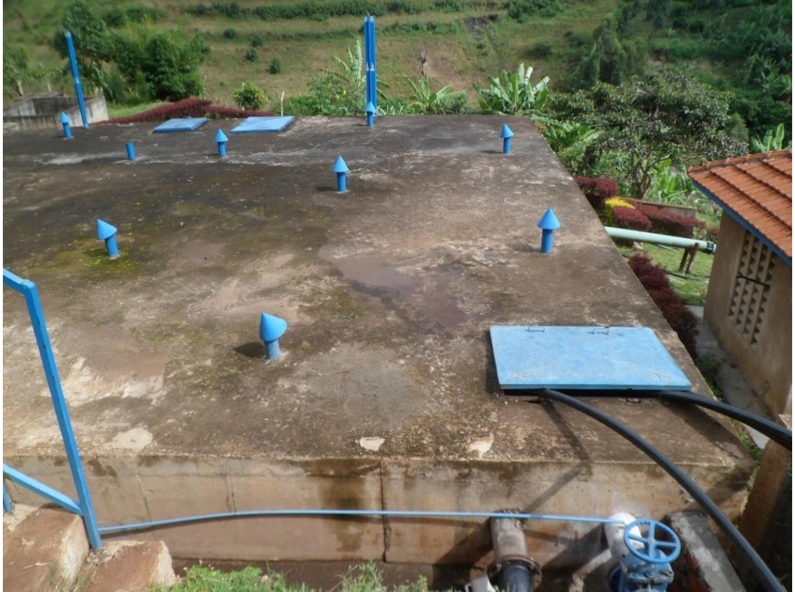
lii) Clear water well with water level meters.
