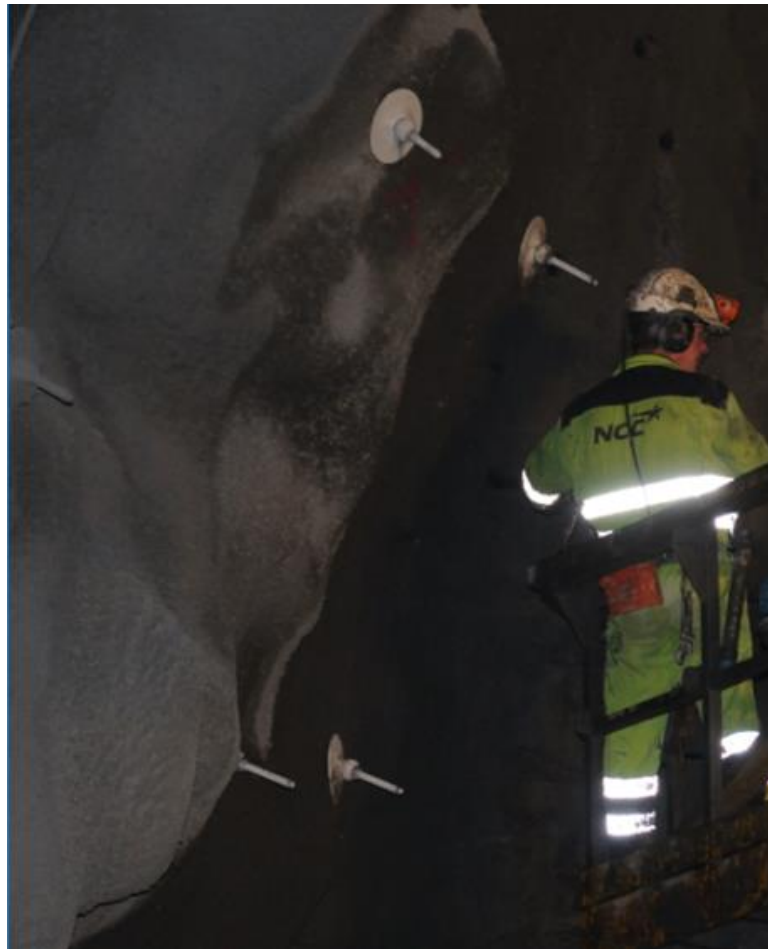
Figure 10-19 : Anchor bolts in Løren Tunnel, Norway
