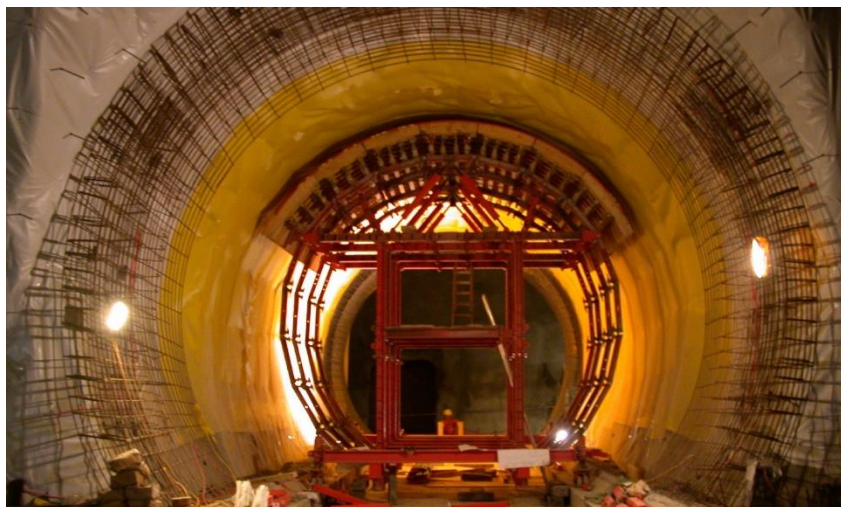
Figure 10-60 : Membrane in place before cast in-situ concrete lining in cross connection, (source Electrowatt Engineering Services)
