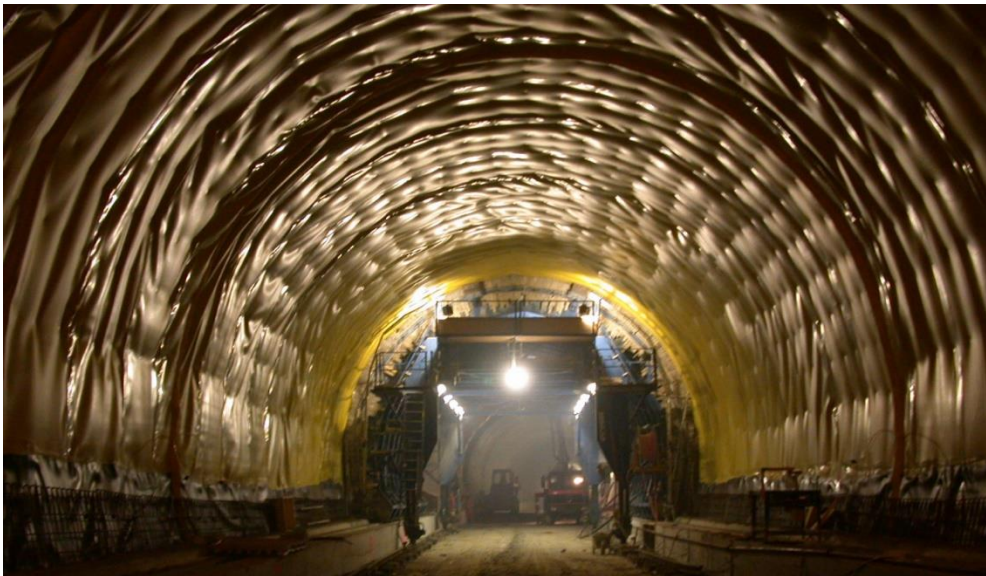
Figure 10-59 : Membrane in place before cast in-situ concrete lining in main tunnel, (source Electrowatt Engineering Services)
