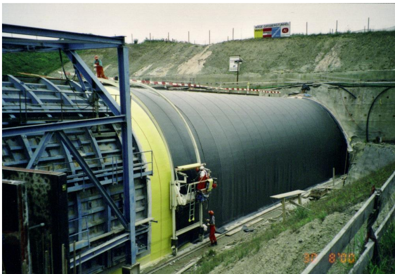
Figure 10-62 : PVC membrane waterproofing for cut and cover tunnel with recycled plastic protection membrane (source ARGE Girsbergtunnel).
