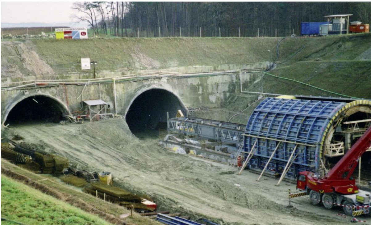
Figure 10-79 : External formwork for cut and cover construction in an open excavation (source ARGE Girsbergtunnel)
