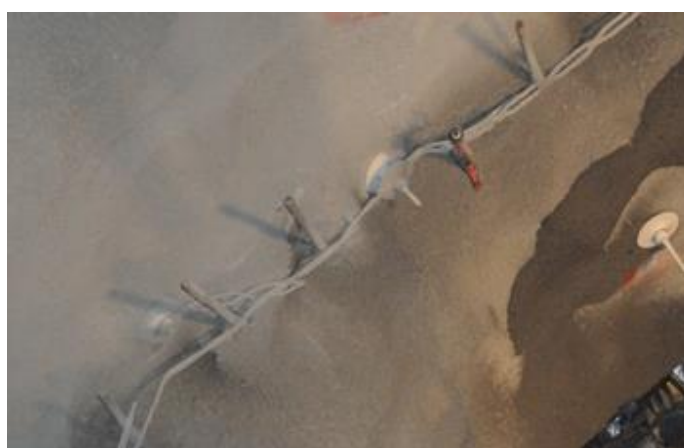
Figure 10-32 : Steel straps in Løren tunnel, Norway
