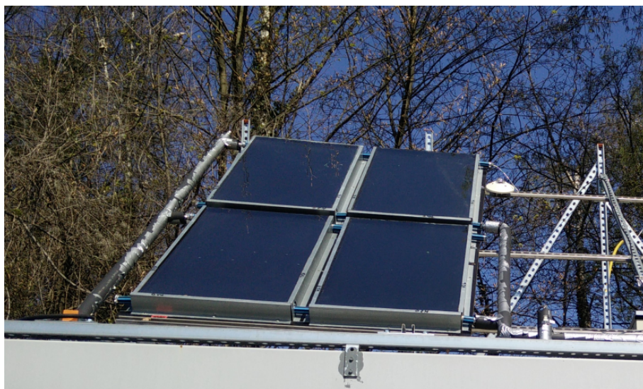
Figure A.3: Collector array. The four polymeric solar thermal FPCs are inclined approximately 5° to the horizontal to ensure a proper self-draining.
