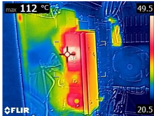
Figure 7.9: Thermal image of the sFCI converter with temperature probing spot on switch S_4 .
