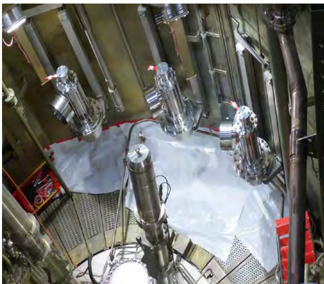
Figure 2: Photo of the three new cooling pumps in the reactor pool of the future ^{99}\text{Mo} -production facility.
