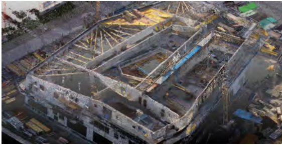
Figure 2. Occluded construction elements in generated point cloud caused by scaffolding, formworks, existing elements and missing information during the reconstruction process
