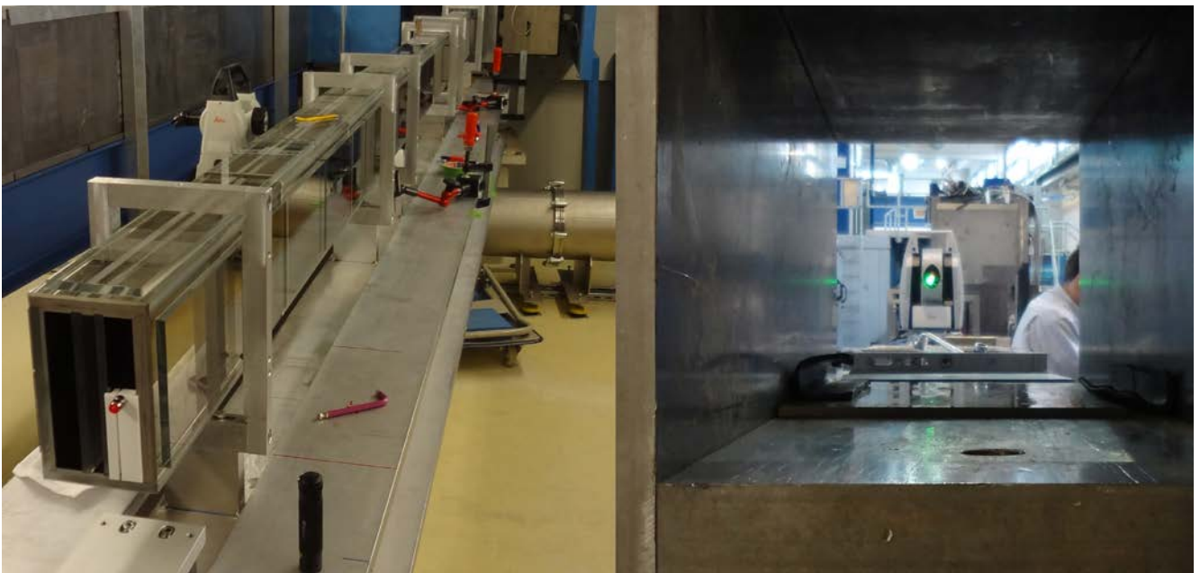
Figure 1: Installation of the neutron guide NL5: the left side shows the first elements of the beam splitter dividing NL5 into NL5-S and NL5-N, while the right side gives a view through the casemate wall into the Neutron Guide Hall West with our Laser Tracker system on the beam line.
