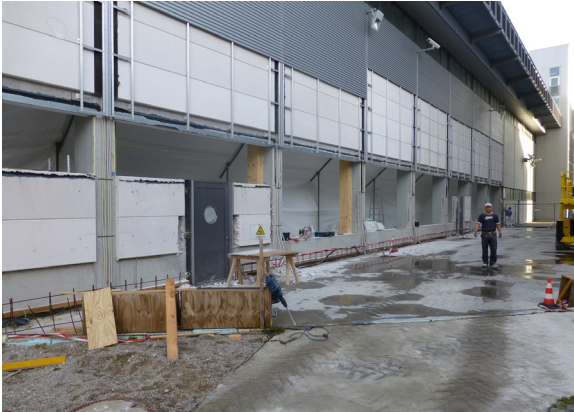
Figure 13: Preparation of the construction zone between the Experimental Hall and the new Neutron Guide Hall East with wall elements already deinstalled.
