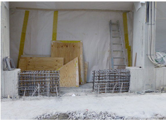
Figure 14: Removal and reconstruction of concrete base for provision of a new entrance from the Neutron Guide Hall East to the new building connecting the Experimental Hall and Neutron Guide Hall East.
