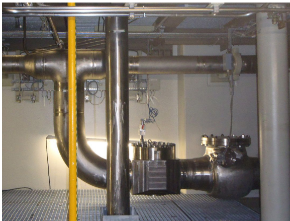
Figure 2: The two main check valves: the new one on the left, the original one on the right.
