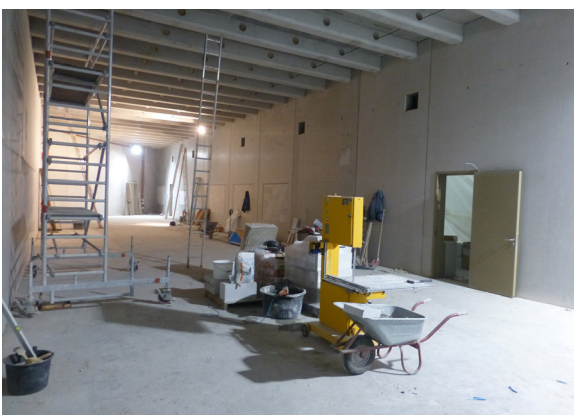
Figure 16: View into the new building connecting the Experimental Hall and Neutron Guide Hall East after concreting work. The new entrance from the Neutron Guide Hall East to the new connecting building can be seen after the access door had been installed (compare to fig. 14).
