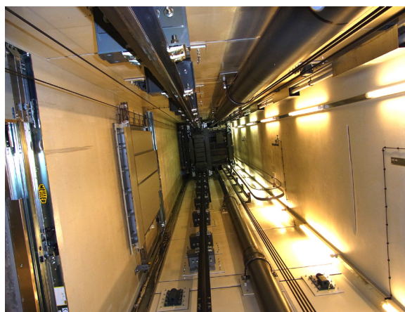
Figure 3: New freight elevator with a lifting capacity of 10 tons in the reactor building.
