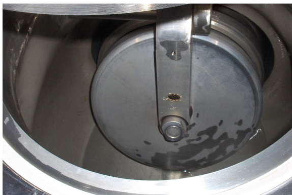
Figure 1: The main check valve to which a second, new one has been added.
