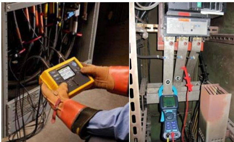
Fig. 8: Power meters to measure the consumption of driving units and whole systems.
