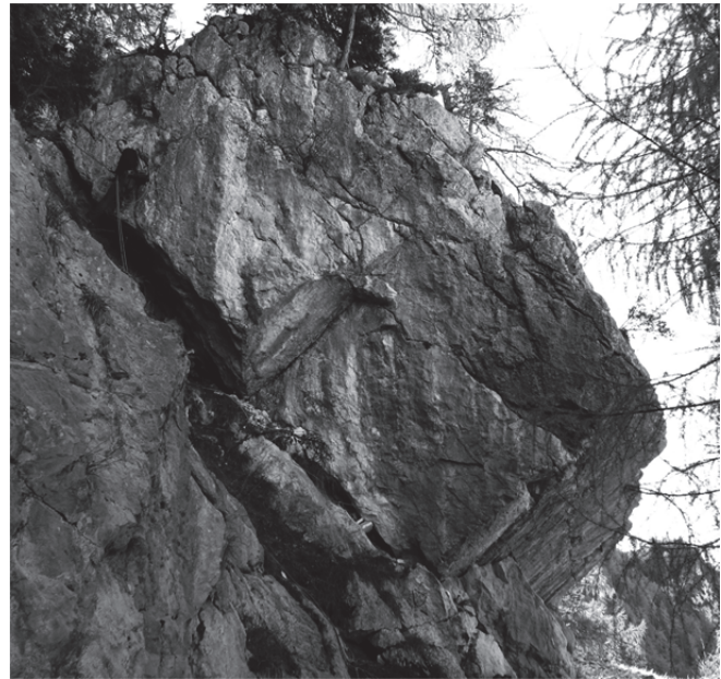
Fig. 1: Block at the release area, a typical example for planar failure. The volume is about 400 m 3 .
