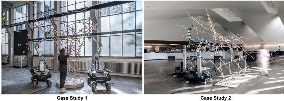
Figure 4.57: Two case studies demonstrating coordinated multi-human-robot cooperative assembly using augmented reality (AR) interfaces. Left: Case Study 1—Turn-taking task distribution for assembling a double-curved funnel structure. Right: Case Study 2—Turn-taking with mobile robotic support for assembling a double-curved shell structure
