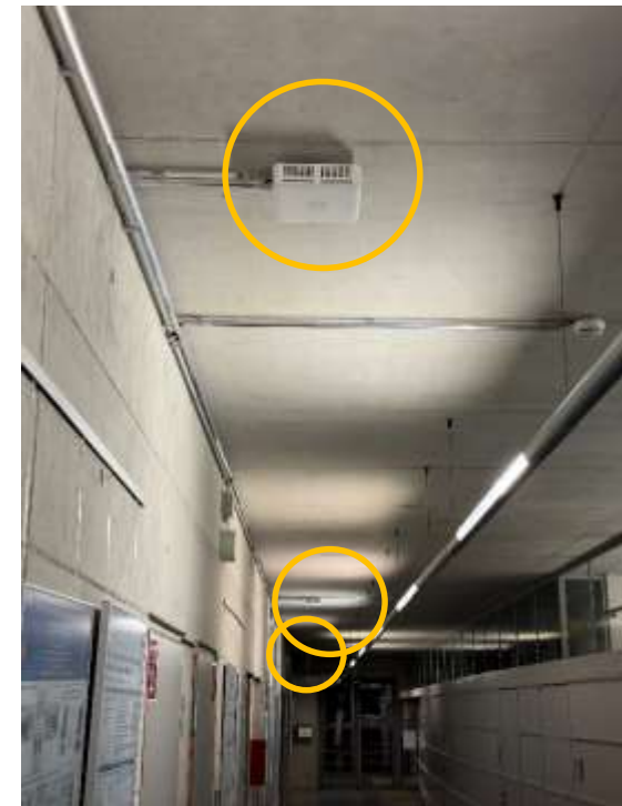
10 indoor base stations
