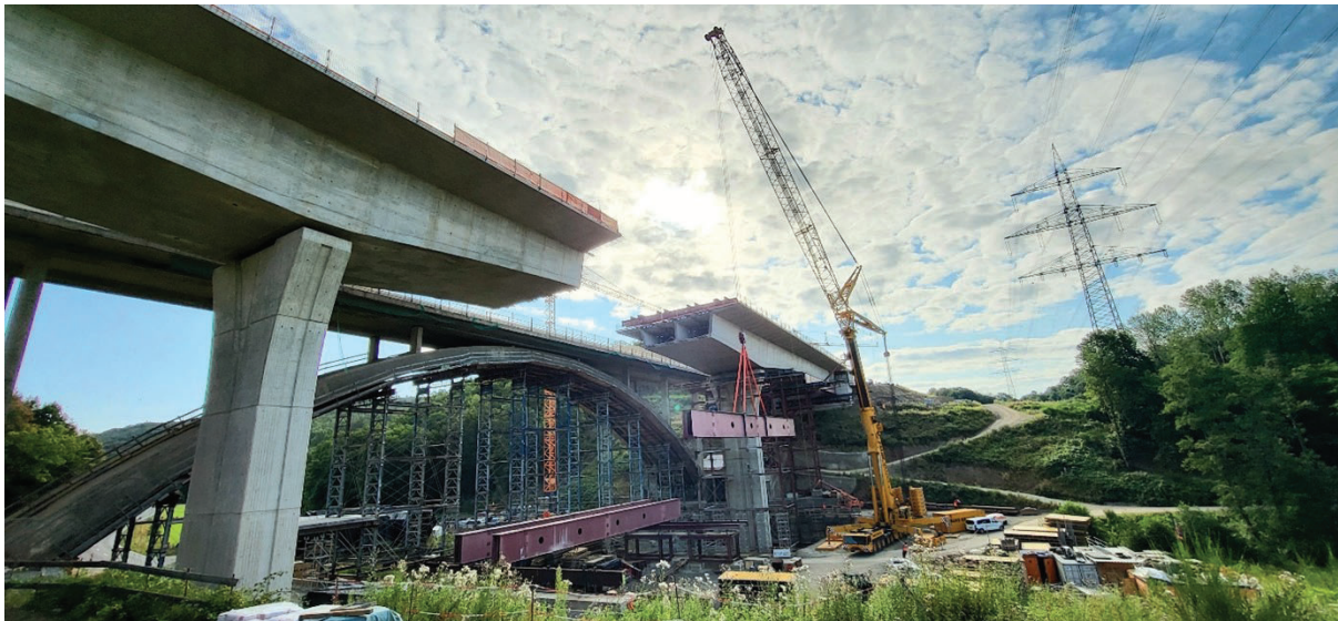
Figure 10: View of BA 1 + BA 2 and preparation of the shoring for construction of BA 3 © Adam Hörnig
