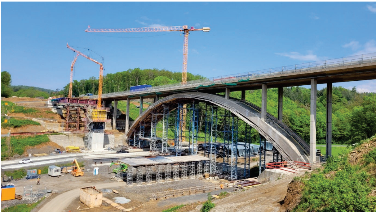
Figure 2: Bechlingen viaduct: Erection of the shoring for the new construction of the substructure for the carriageway in the direction Hanau and the existing arch bridge of the substructure for the carriageway in the direction Dortmund © Adam Hörnig
