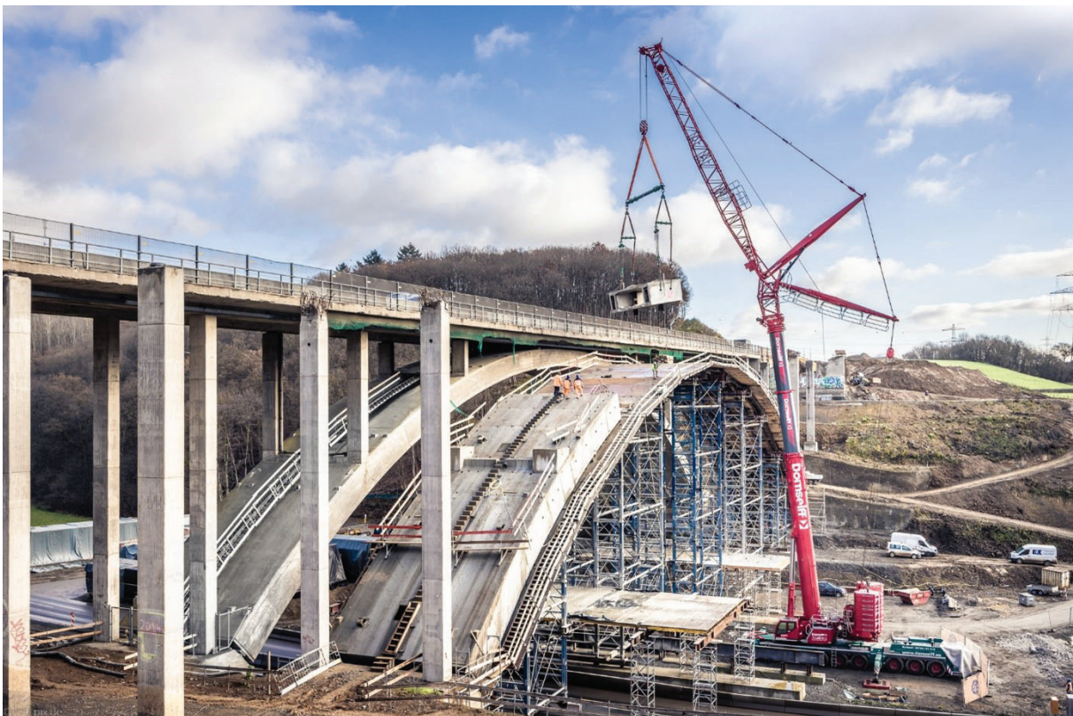
Figure 4: Lifting out the cut-out arch elements using a mobile crane © Adam Hoernig
