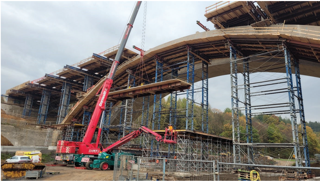
Figure 3: Demolition of the existing structure: demolition support scaffolding and excavation of the carriageway slab elements © Adam Hoernig
