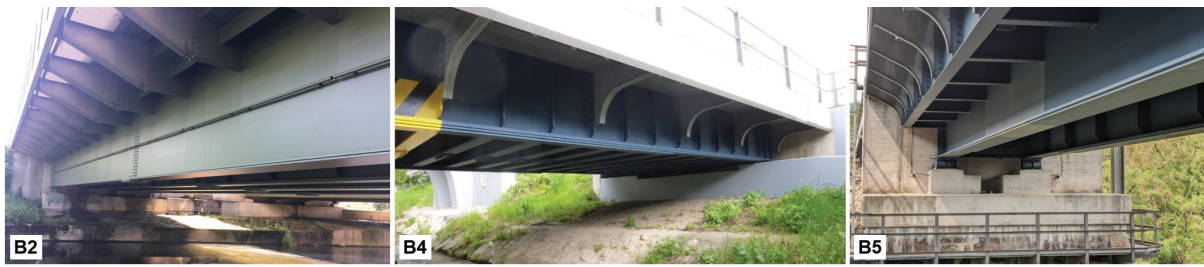
Figure 5: Exemplary overview of three selected bridges of the measurement campaign (B2, B4 and B5)
