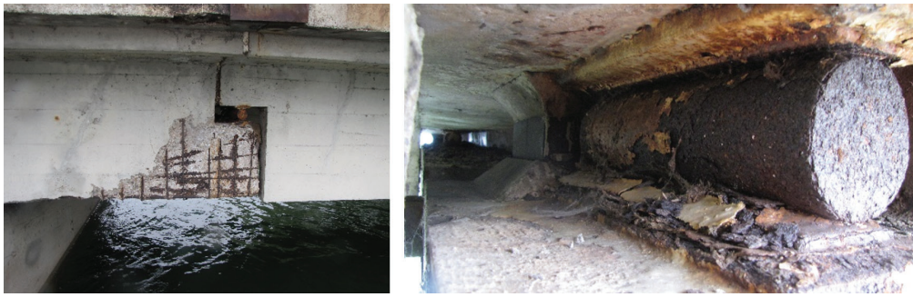
Figure 3: Strongly corroded reinforcement at the girders (left); Detail: corroded bearing between two girders (right)
