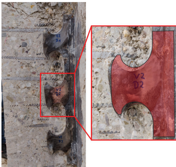
Figure 5: Deformation of steel teeth in static test of upper part
