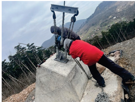
Figure 17: Connecting the individually fixed windties at the starting sections of the bridge
