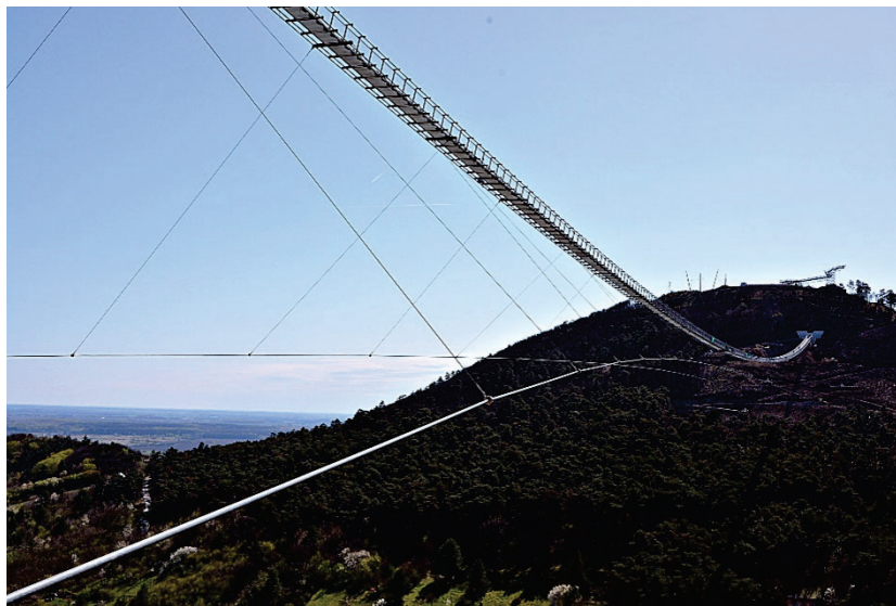
Figure 6: Wind cable system
