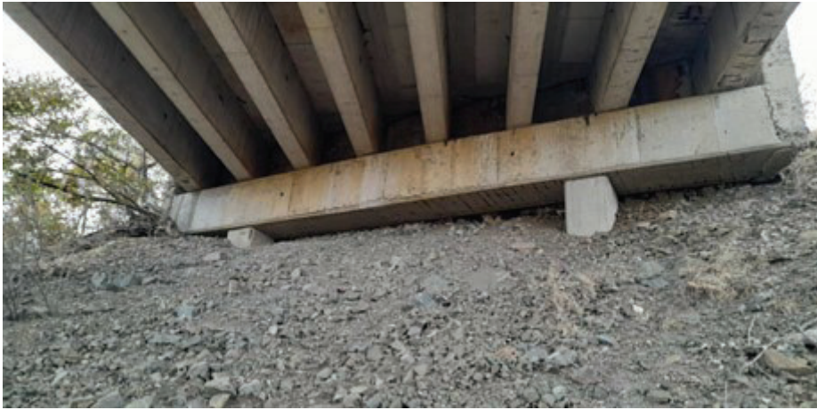
Figure 7: An example of damage to the embankments at an open-end abutment
