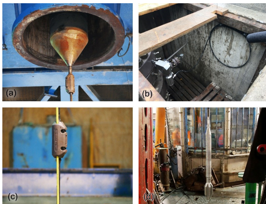
Figure 5-2. Installation of the FO-cable in the producer well. (a): \frac{3}{4} inch to 1\frac{3}{8} -in. crossover. (b): Wellhead outlet. (c): TEF mounted on sucker rods with clamps. (d): Carrier at termination with centralizer.
