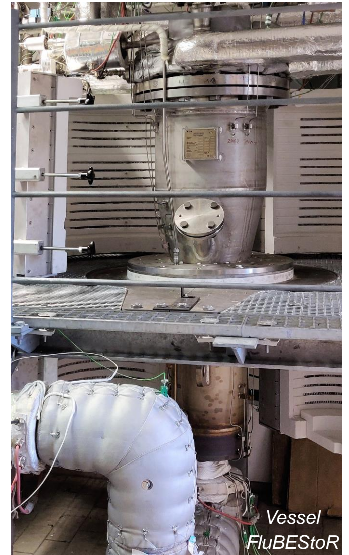
Vessel and Peripheries FluBEStoR
