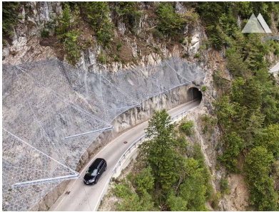
(a) Angled rock fall protection structure, spanning over a road (Route Chalais-Vercorin, Valais). Source: Geobruigg www.geobruigg.com
