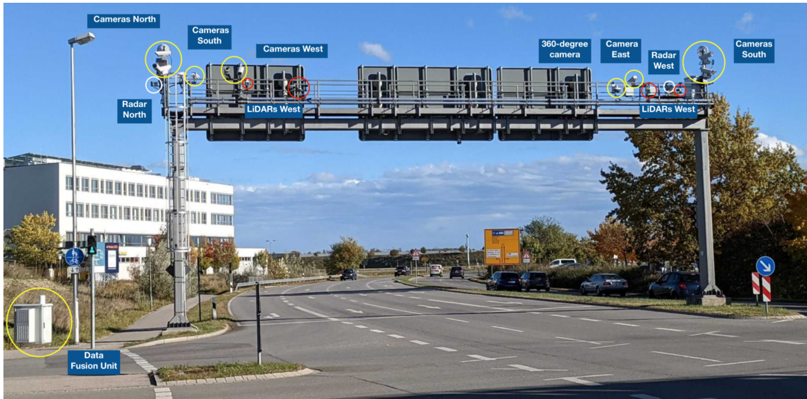
Figure 2.5: Equipped gantry bridge near Munich, Germany as part of the Providentia++ project.
