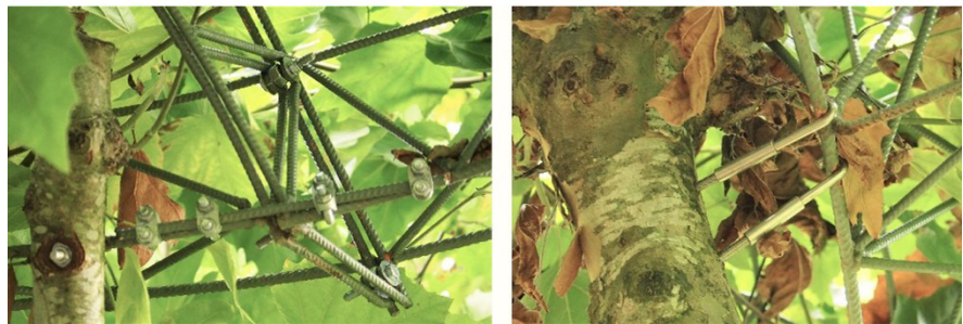
Figure 3: Detailed connection techniques. Left: truss pieces were connected by M8 screws, reinforced with rebar stick and metal rings. Right: the space frame was fixed to trees with screw hooks.
