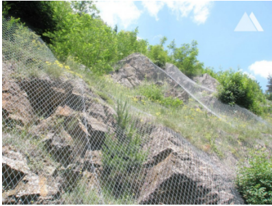
(a) Banya railway rockfall protection, active.
