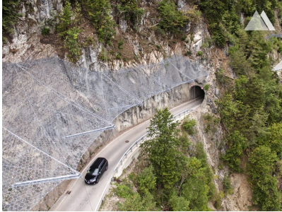
(a) Route Chalais-Vercorin, Valais. Photograph is property of Geobruigg ( https://www.geobruigg.com ).
