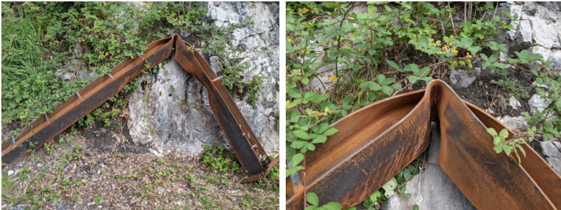
(a) Column with plastic damage.
