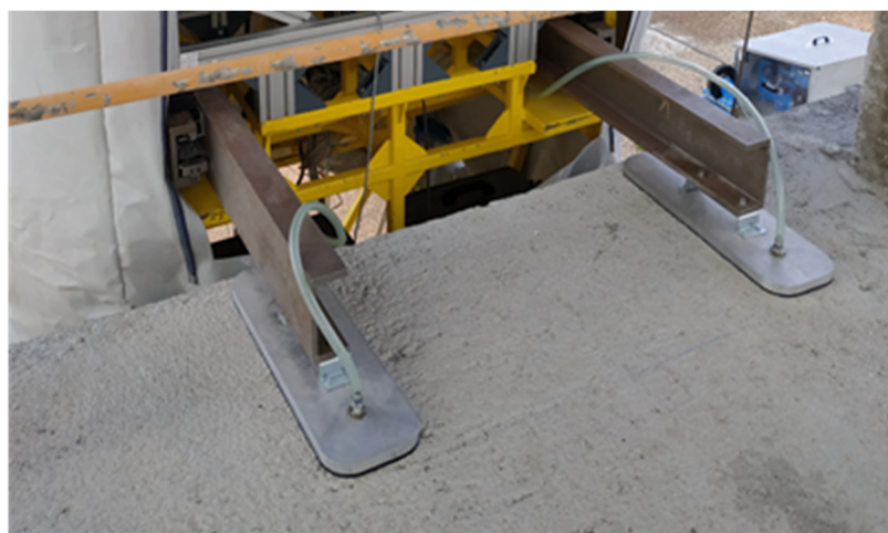
Figure 8. Stabilizer attaching the robot platform to the concrete slab (photo: José David Jiménez-Vicaría).
