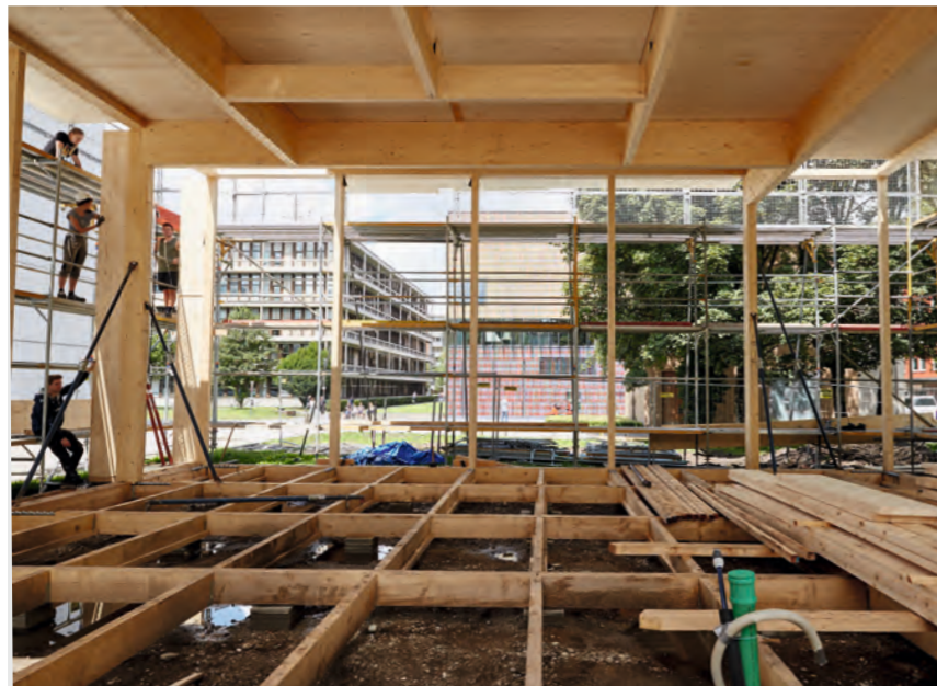
Students and supervisors spent much time on the construction site during the summer of 2020.
