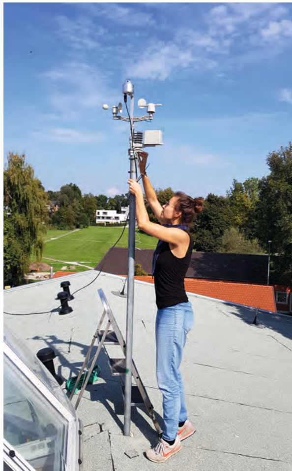
Fig. 2. Installation of the weather station on the roof of the lightweight concrete house. Photo: TUM staff
