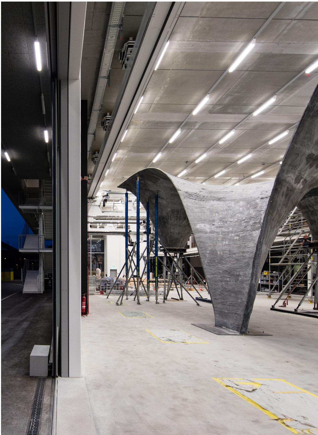
Professur Philippe BLOCK: Ultra- thin, curved concrete roof as part of a roof- top apartment unit called HiLo (NEST project)
