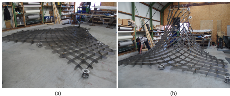
Figure 7.17: Mounting process of the canopy grid in the workshop: (a) flat assembly on the ground and (b) intermediate state during the mounting.
