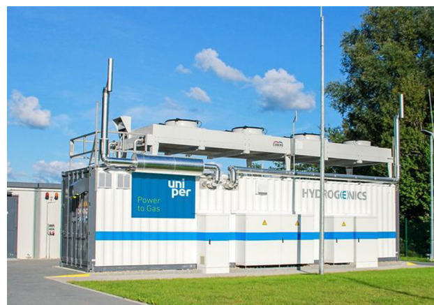
Fig. 4. Typical containerized PEMWE system in the 1 MW power range at Windgas Hamburg, Reitbrook project site. (Copyright ©Uniper SE).
