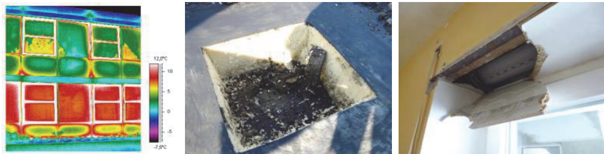
Figure 4 Thermal image, open roof membrane (wet insulation), window shutter
