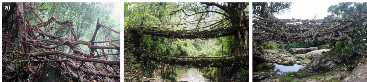
Figure 6. (a) Partial view of Siej bridge (#50). The bridge is an example of bridges that are grown by currently living people. (b) According to the statement of residents/users involved in the maintenance the bridge in Nongriat village (#6) is estimated to be ca. 200 years old, an example of bridges started by known ancestors. (c) The bridge linking the two sides of Nongbareh village (#62) is part of a vital route. It is estimated to be as old as the village, probably hundreds of years old.
