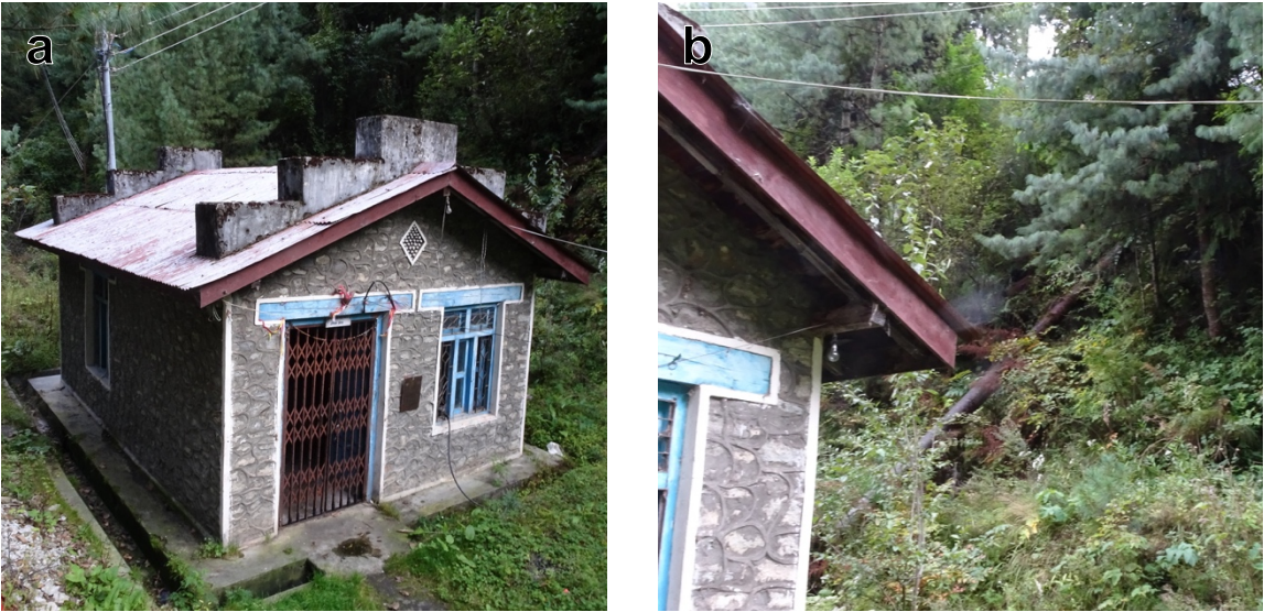
Figure 2-11: Powerhouse (a) and penstock (b) of Chame Hydropower Plant [Own Illustrations]
