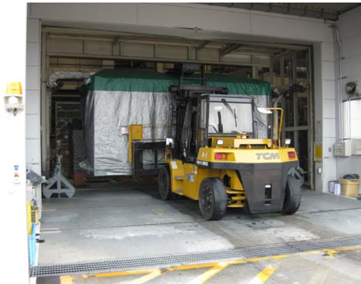
Figure 10: At the last workstation within the factory, the finished modules are prepared for transport.
