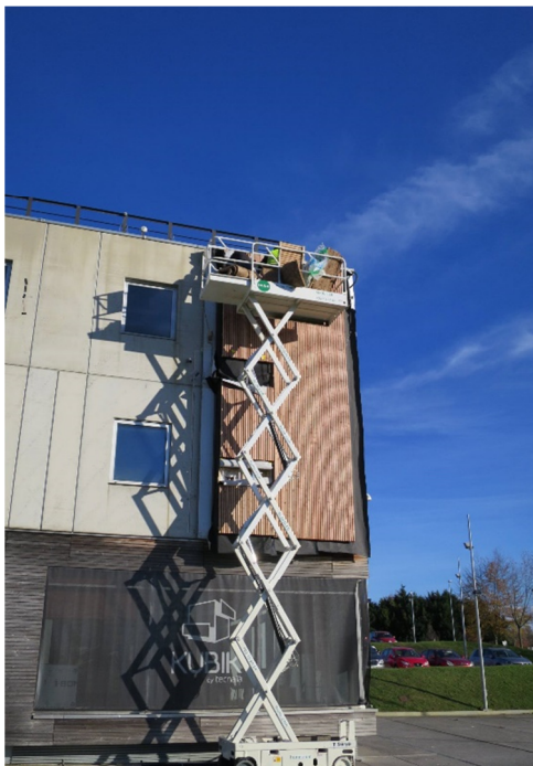
Figure 4: BERTIM facade modules installation in one of the sites (Image: M. Eng. Kepa Iturralde).
