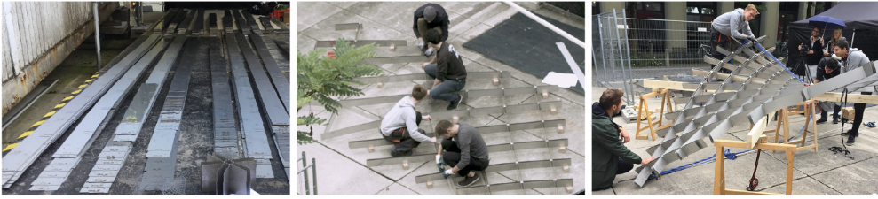
Figure 14: The straight lamellas are interlocked by hand into flat segments. The segments are then transformed elastically into their designed shape. This erection process follows a compliant mechanism, without the need for scaffolding. Nine of these segments were prefabricated off site.
