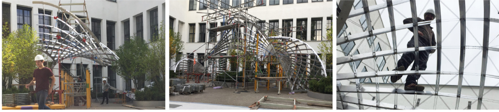
Figure 15: Installation on site. The prefabricated segments of up to 400 kg, were positioned with a crane, temporarily supported, and bolted together by hand. To activate the structural behavior of a gridshell, the completed grid is braced diagonally and fixed at supports in vertical and horizontal direction.
