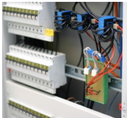
Figure 6.0.1: CAT-6 cables to transfer power and current data
