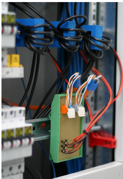
Figure 6.2.3: CLEAR current sensors installed in the electric cabinet. The open-loop Hall-effect sensors employ multiple turns of the mains wiring to increase the usable output signal. A small connection board distributes supply voltage and output signals. All changes and alterations were authorized and conducted by certified personnel.
