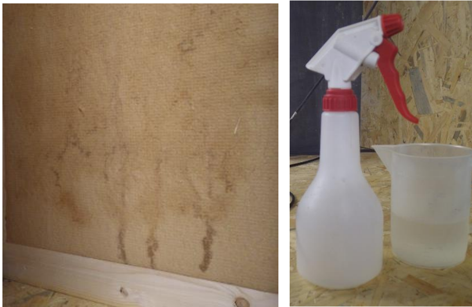
Figure 50. Wood fiber board had water stains after spray test.
