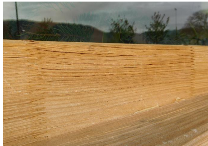
Figure 20 Deformation of a window frame - FCBA expertise.
