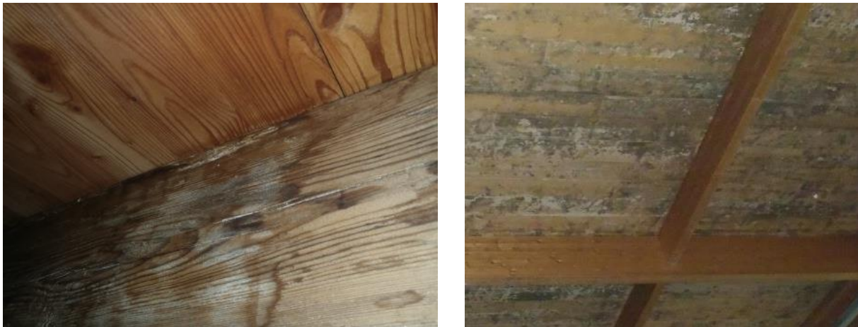
Figure 17 Indoor facing with traces of mold – FCBA expertise.
