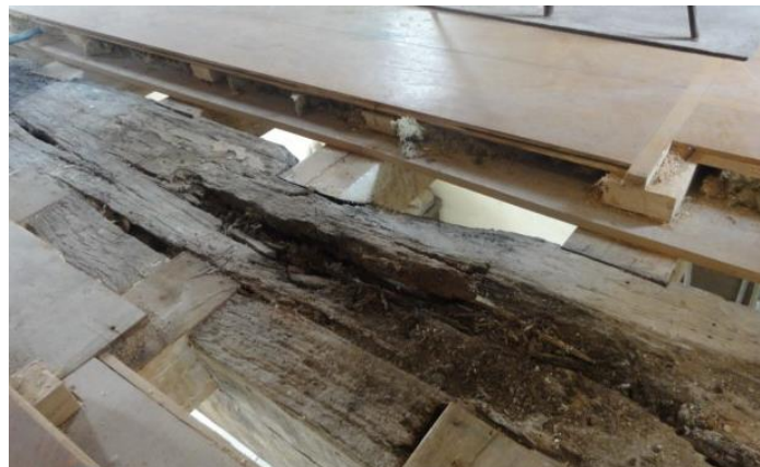
Figure 16 Illustration of a damaged floor structure - FCBA expertise.
