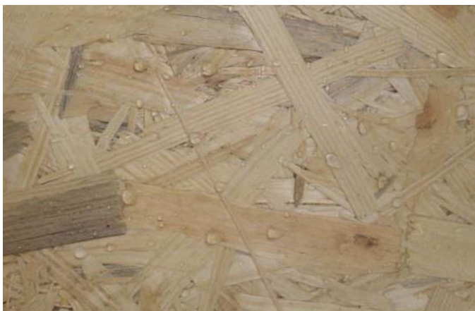
Figure 64. OSB panel surface after watering the interior face showed water drops and poor hygroscopic behavior
