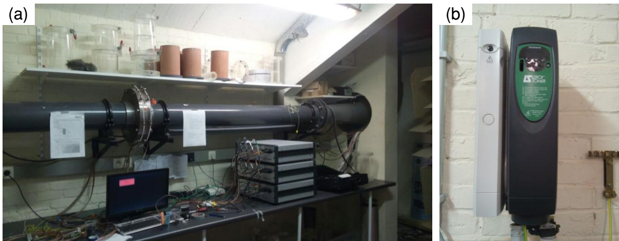
Figure 3.2: (a) Acoustic mufflers connecting the blower to the anechoic chamber. (b) Electronic control unit of the blower.
